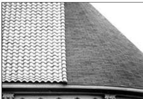
Asphalt shingles are an incompatible replacement substitute for the original Spanish clay tiles. Photo: NPS files.
