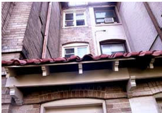
An eave closure or birdstop to keep out birds is notably absent from the replacement tile in the center of the bottom row. Photo: NPS files.
