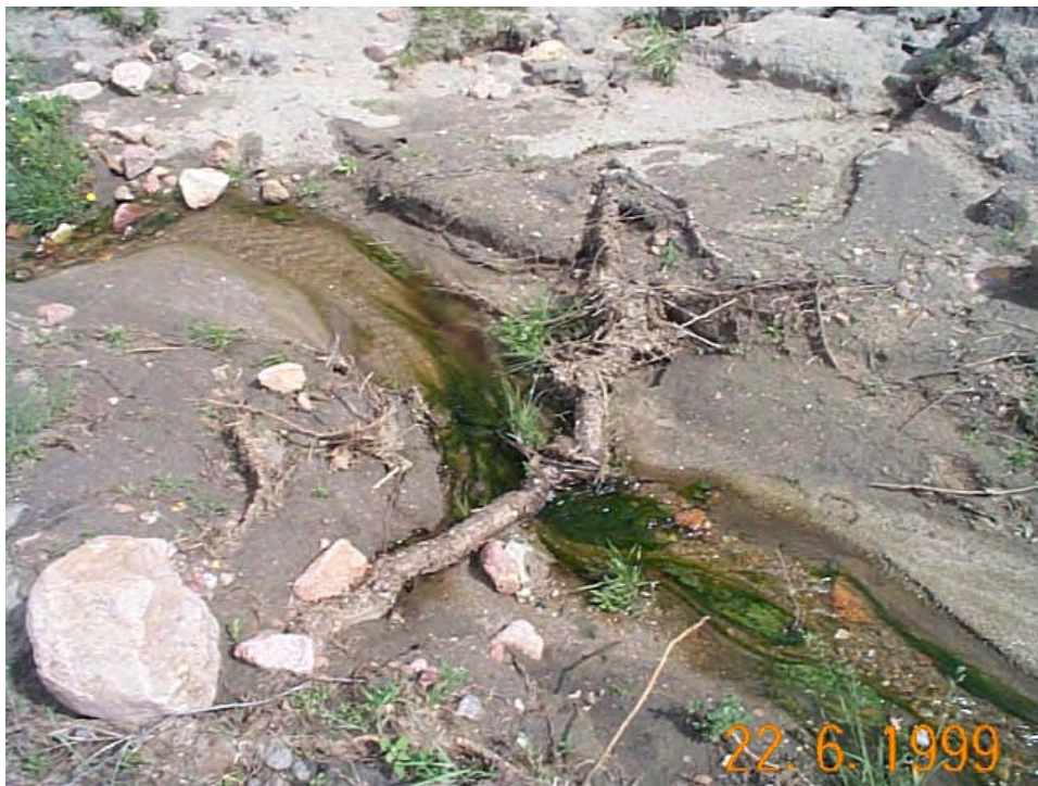
Figure 9. Large pine tree root located in the channel of the breach opening of a failed Air Force Academy waste lagoon pond dam (David Eyre, Senior Civil Engineer, Air Force Academy, Colorado, 1999).
