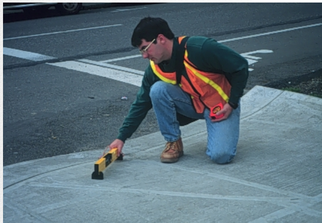
Figure 11-1. Collecting objective information about sidewalk conditions is a critical step towards improving the accessibility of existing pedestrian networks.
