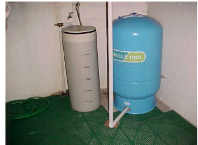
A Hydropneumatic Storage Tank
