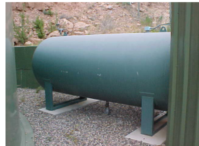
A Metal Storage Tank
