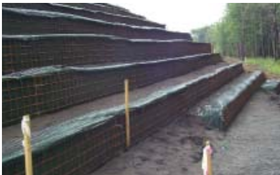
Figure 12. Stepped embankment (Ohio turnpike, sand supplied by Kurtz Bros. Inc., construction by Trumbull Corp.)
