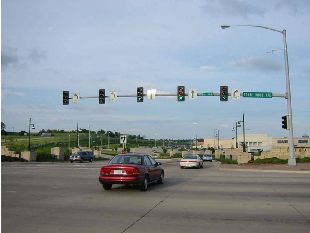
Figure 114. Lane-aligned signal heads.
