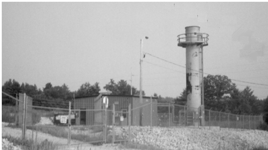
Figure 5-7. Enclosed Ground Flare and Blower Station.
