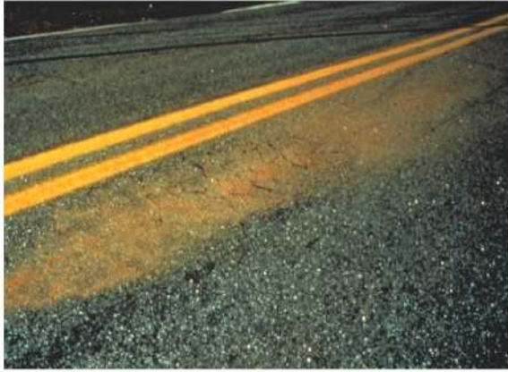
c) Subgrade pumping
