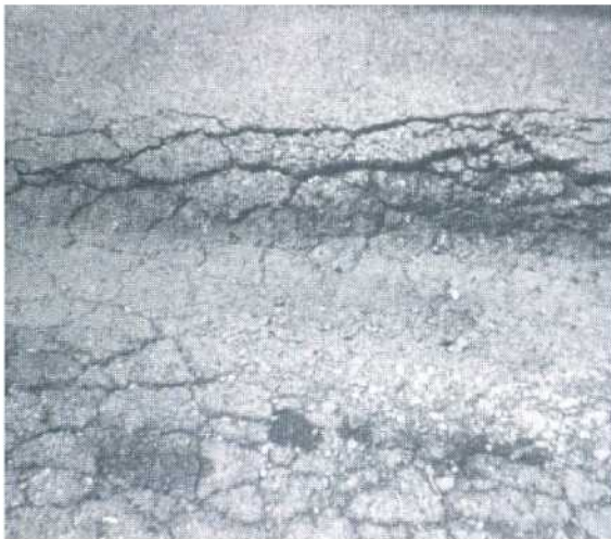
a) Excessive rutting
