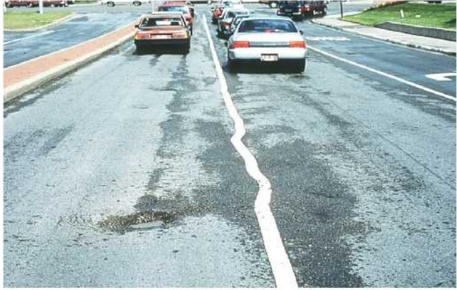
d) Drainage problems
