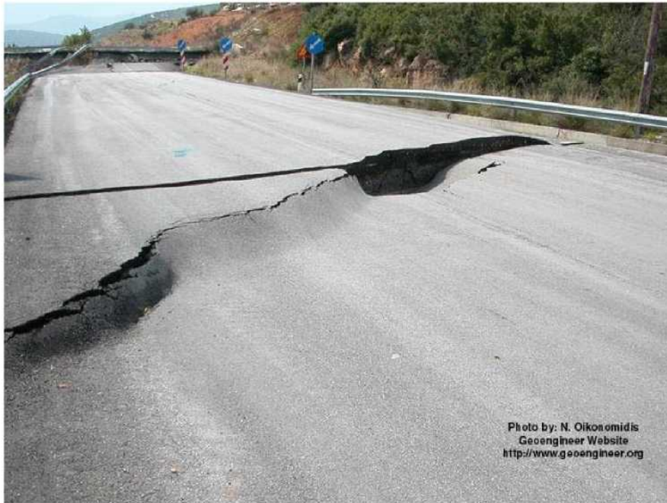
Figure 3-7. Slope failure beneath road pavement (www.geoengineer.com).
