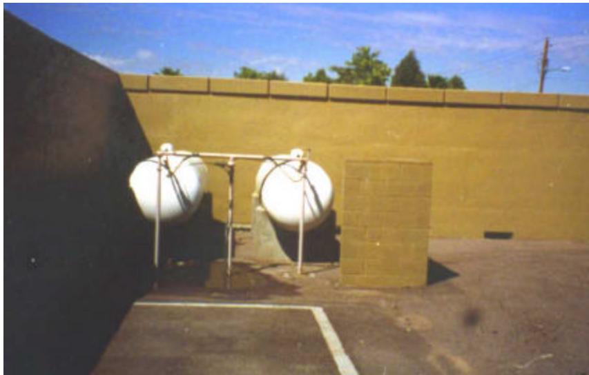
Figure 11-1. Liquid propane tanks for pump station power
