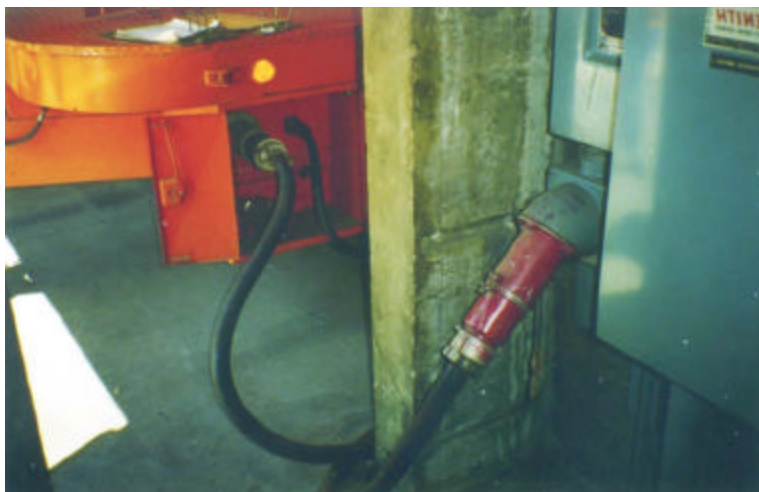
Figure 11-5. Mobile generator and standby power receptacle
