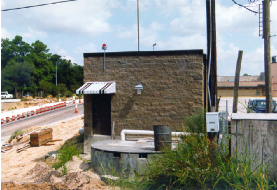
Figure 3-9. Small pump house for vertical pumps in Houston, Texas
