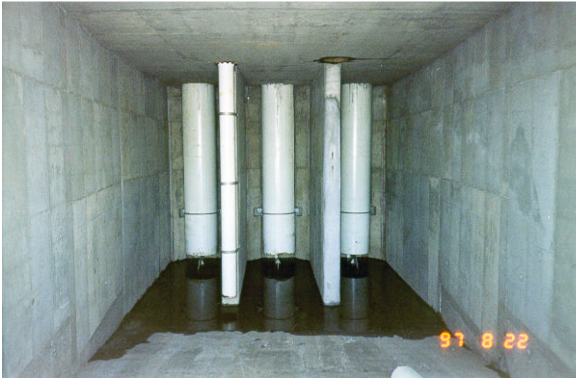
Figure 3-10. Rectangular pit with submersible pumps
