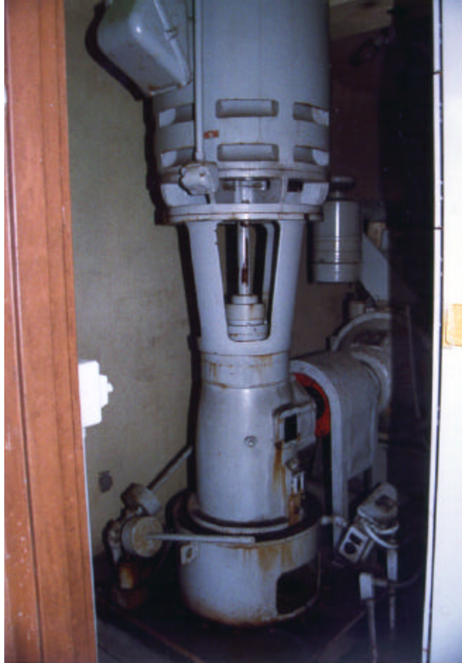
Figure 13-1. Old motor drive for vertical pump to be replaced
