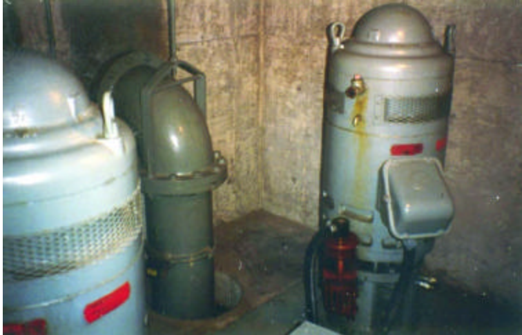
Figure 11-2. Typical electric motors for vertical pumps
