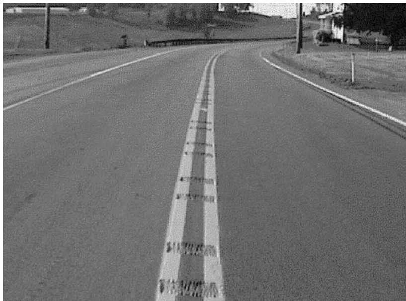
EXHIBIT V-5 Centerline Rumble Strips (Photo Provided by PennDOT)
