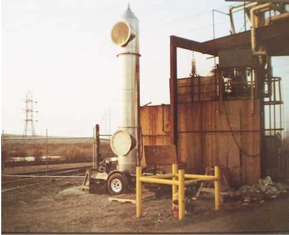
Figure 10 Photograph of a typical operating mobile packed column air stripper
