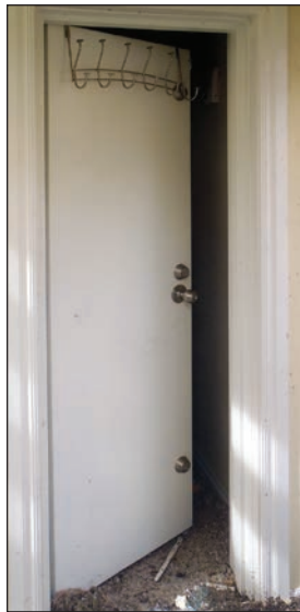
Residential safe room door (Moore, OK, 2013)
