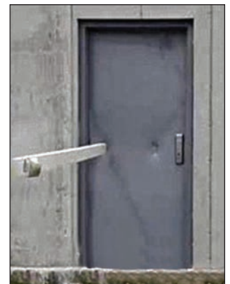
Tornado safe room impact test results: Door assembly passed; no perforation or latch/lock failure
