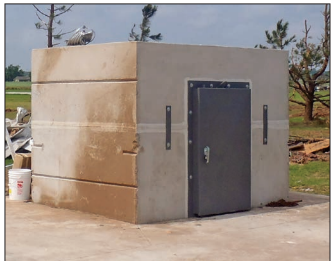
Figure 5-1: Safe room that remained standing after an EF5 tornado (Newcastle, OK, 2013). The photo shows the safe room after the event, after debris had been cleared away.
