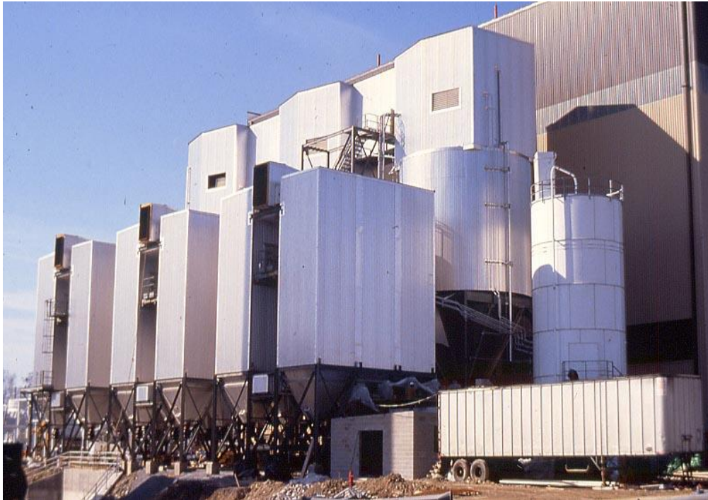
Fig. 7 Spray Dryer Absorber System on WTE Plant
