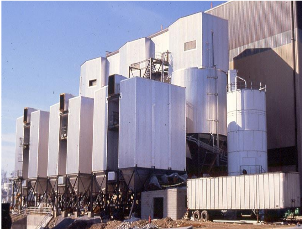
Figure 6. Spray Dry Absorber System for Acid Gas Control
