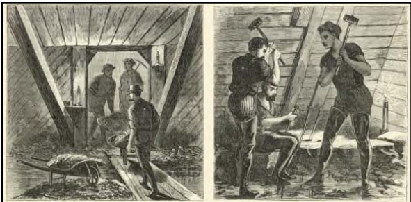
Left: Workman passing a wheelbarrow full of “spoil” through an opening in a support frame Right: Workmen using a Sisyphus and sledge hammers to break boulders
