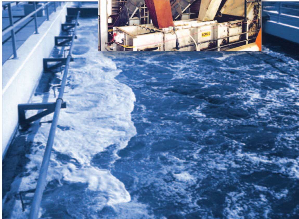
Aerated Grit Chamber
