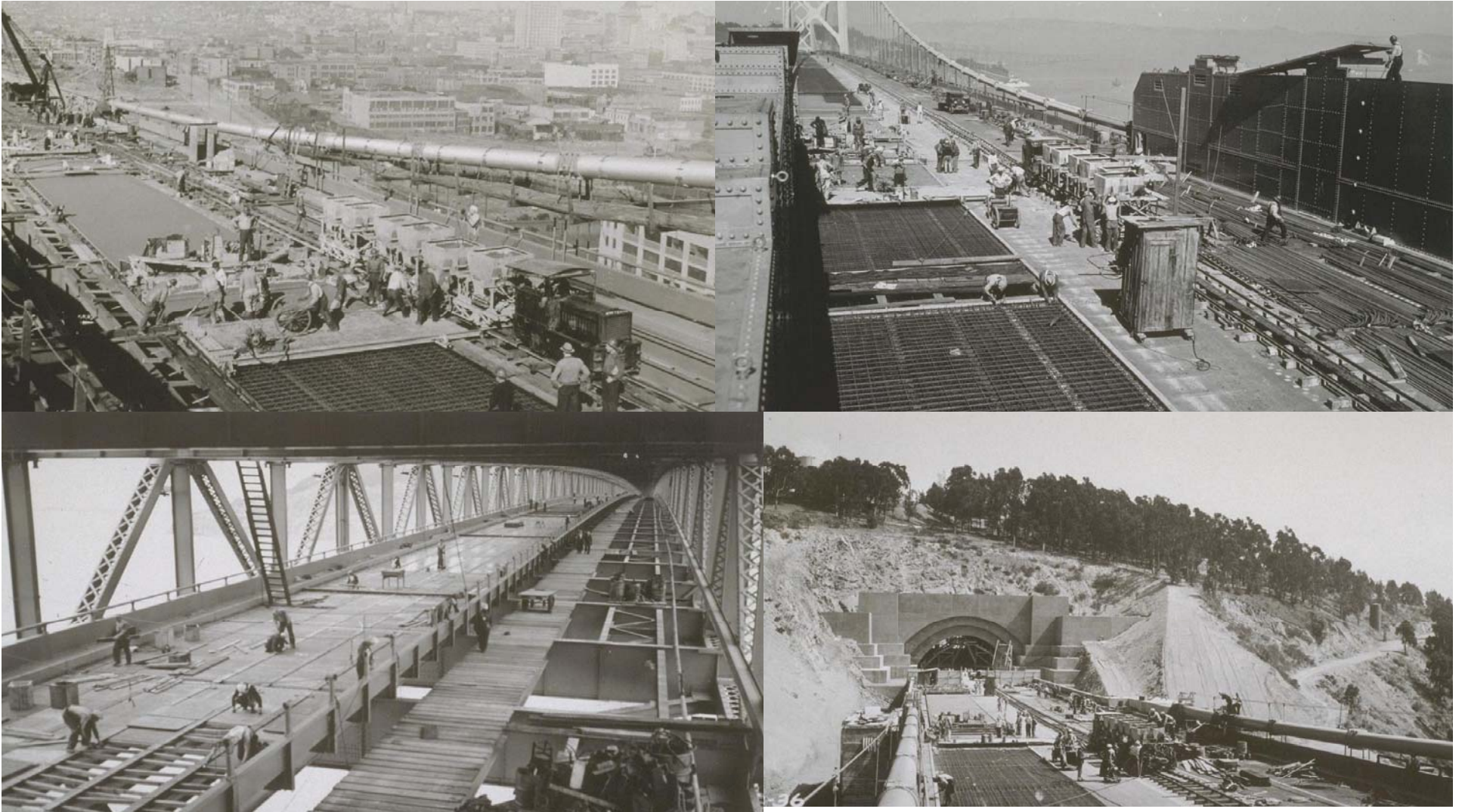
Upper Left – suspension-span upper deck (between W-2 and W-3) Upper Right – suspension-span upper deck (Central Anchorage) Lower Left – suspension-span lower deck (between W-5 and W-6) Lower Right – suspension-span upper deck (Y-B Anchorage) 410
