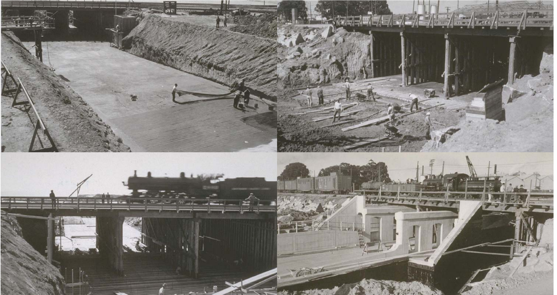
Folger Avenue Underpass (Contract No. 42) Upper Left/Right – August 1935 Lower Left – August 1935 / Lower Right – Nov. 1935
