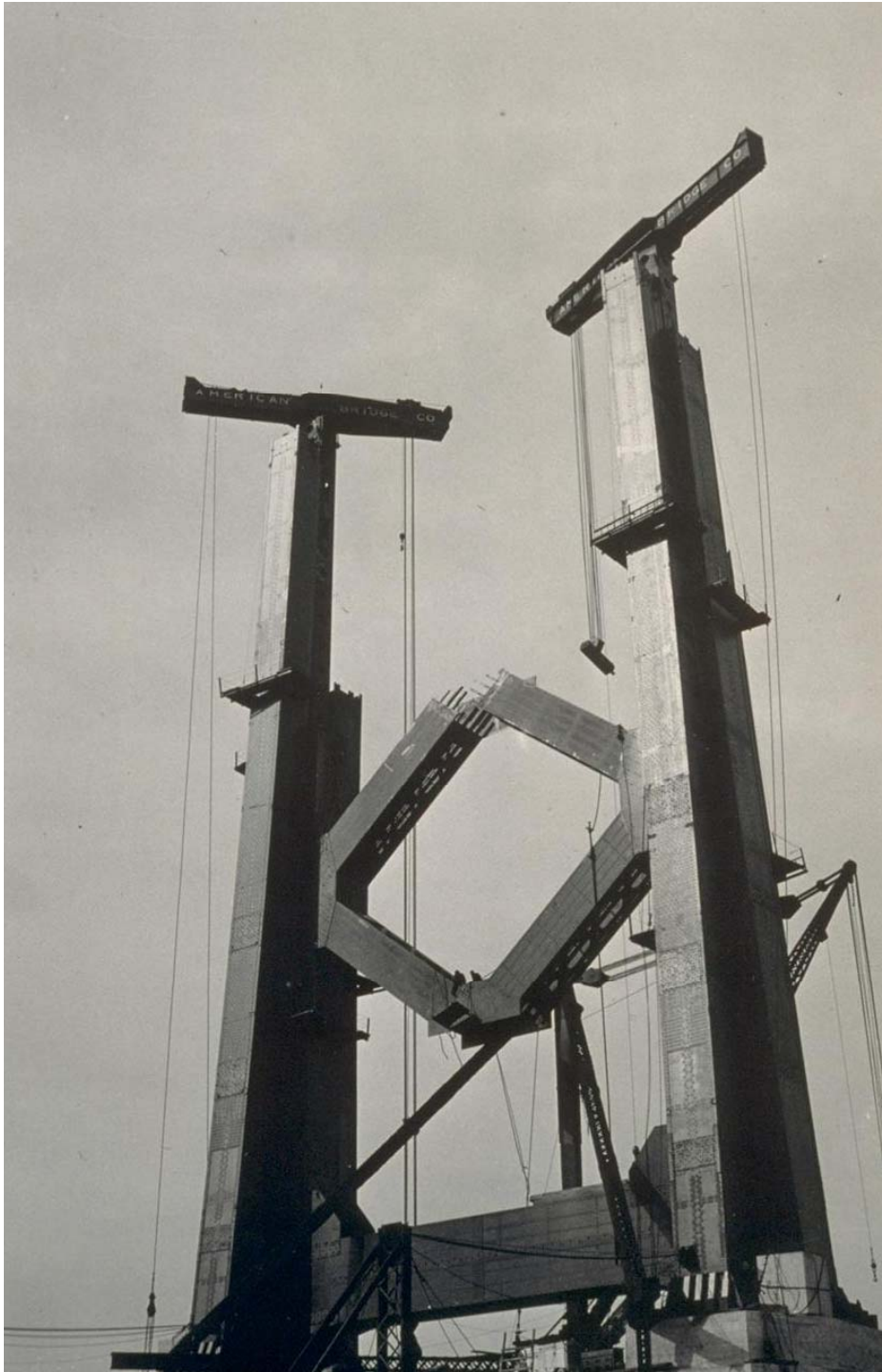
Tower No. 2 Horizontal Base Strut in position and X-Bracing being erected (April 1934)
