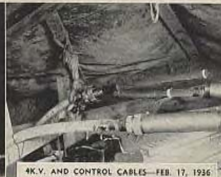
4K.V. AND CONTROL CABLES—FEB. 17, 1936
