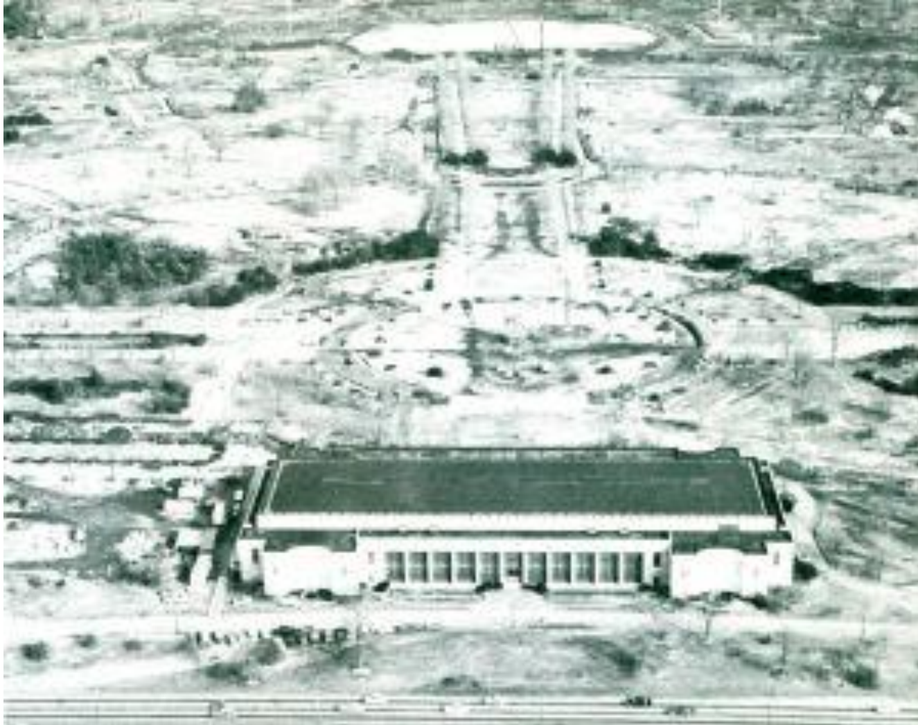
Construction of utilities and roads at the site of Unisphere and along the Main Mall. City of New York Building (from the 1939/40 NYWF) and Grand Central Parkway in foreground.
