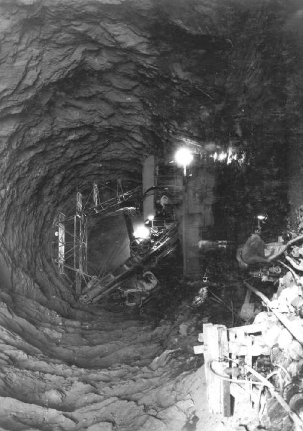
Excavating invert material near outlet portal of Arizona Penstock tunnel. View looking upstream (February 1932).
