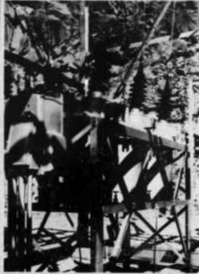
CIRCUIT BREAKERS IN BOULDER CITY SUBSTATION
