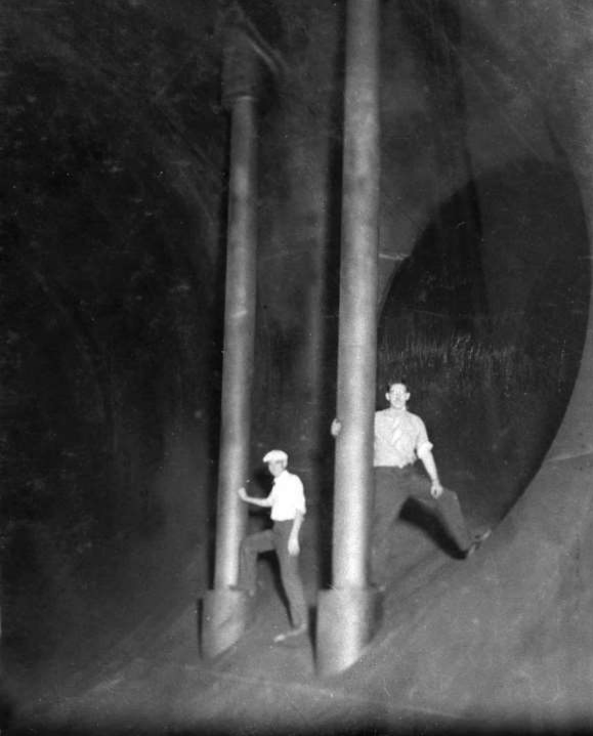
“T-section” of Penstock pipe where thirty-foot section branches to 13-foot section leading to Nevada wing of Powerhouse (note stiffener shafts; May 1936)
