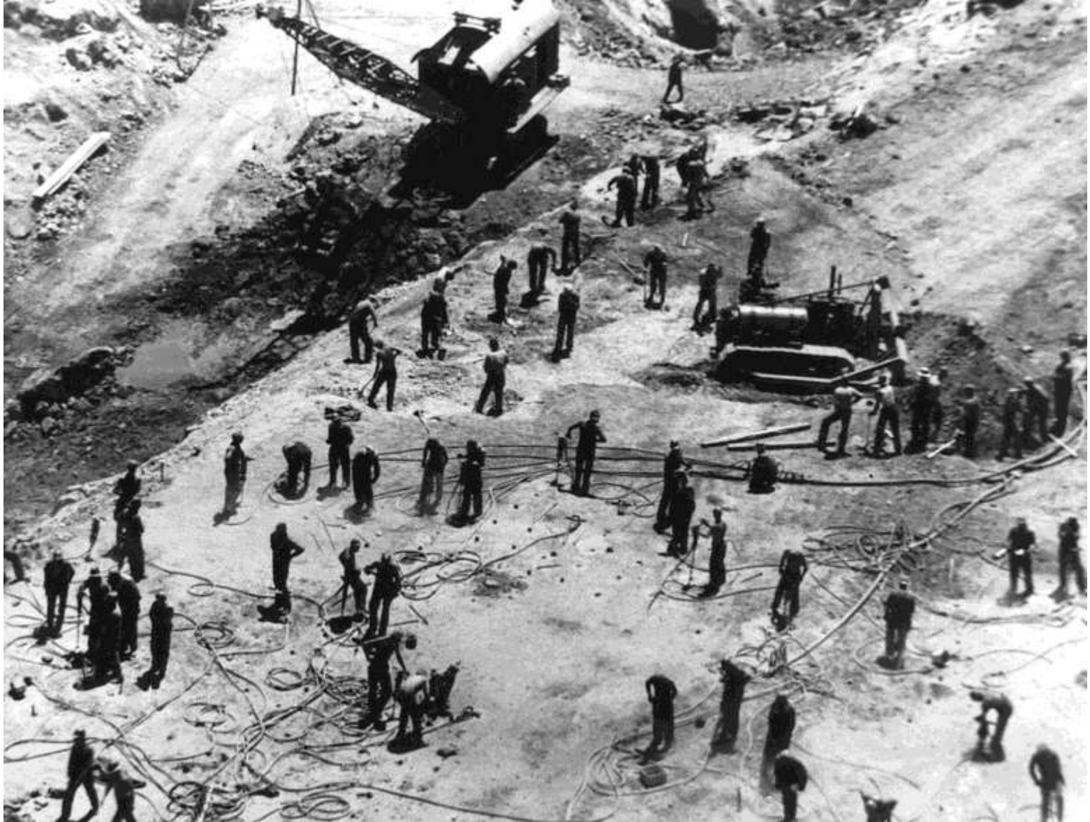
Drill crews on the Nevada bench of the dam foundation excavation. Fifty-six drills were in operation in this relatively small area (June 1933). 542
