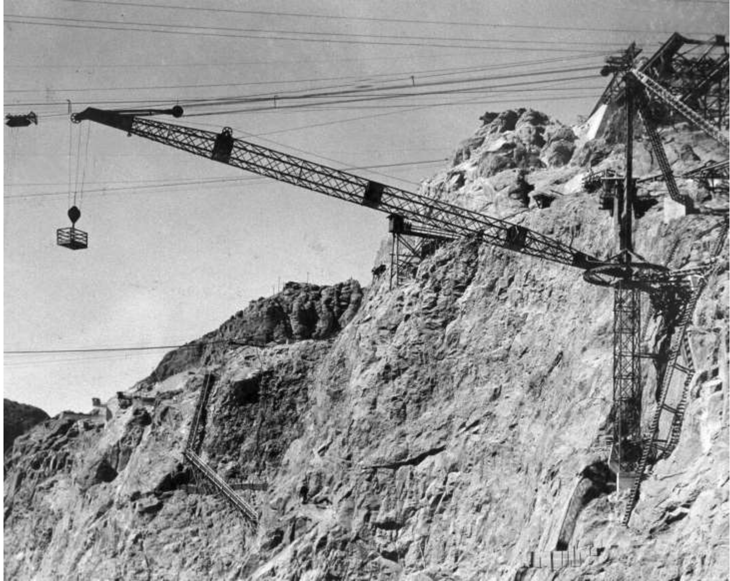
Twelve-ton capacity crane erected by Six Companies to handle concrete and materials for Nevada Intake Towers and outlet raises (September 1933)
