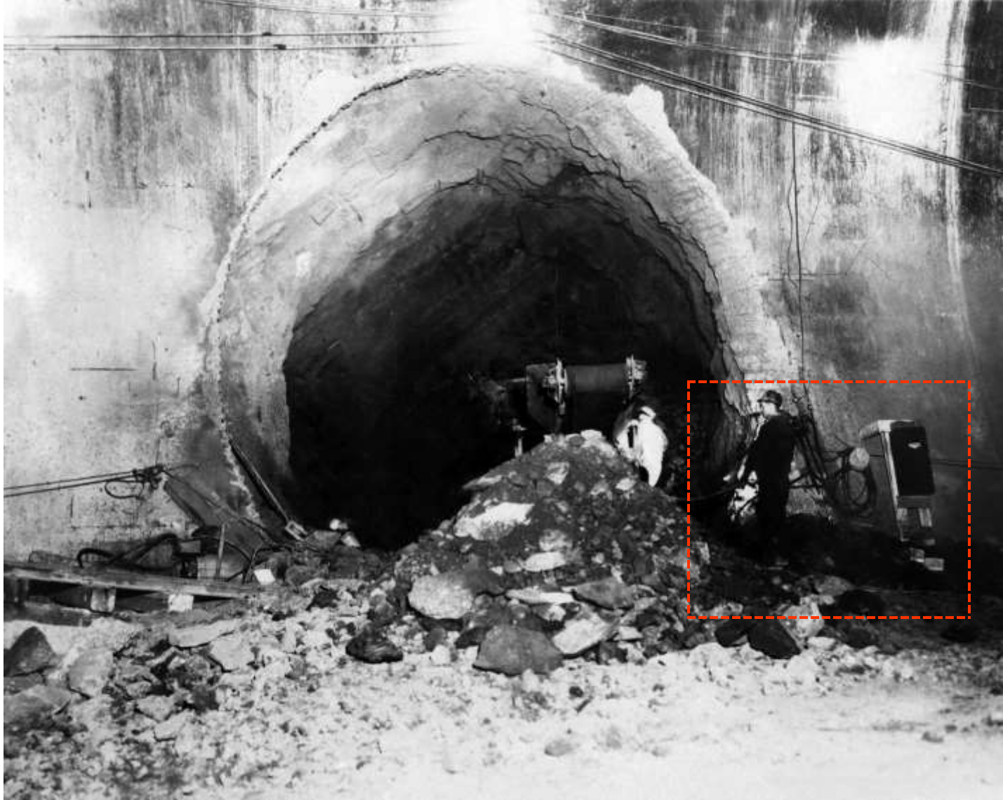
Start of operations on driving of 18-foot Penstock Adits (from Diversion Tunnel No. 2) to Nevada Powerhouse (showing Conway Mucking Machine removing muck; December 1932).
