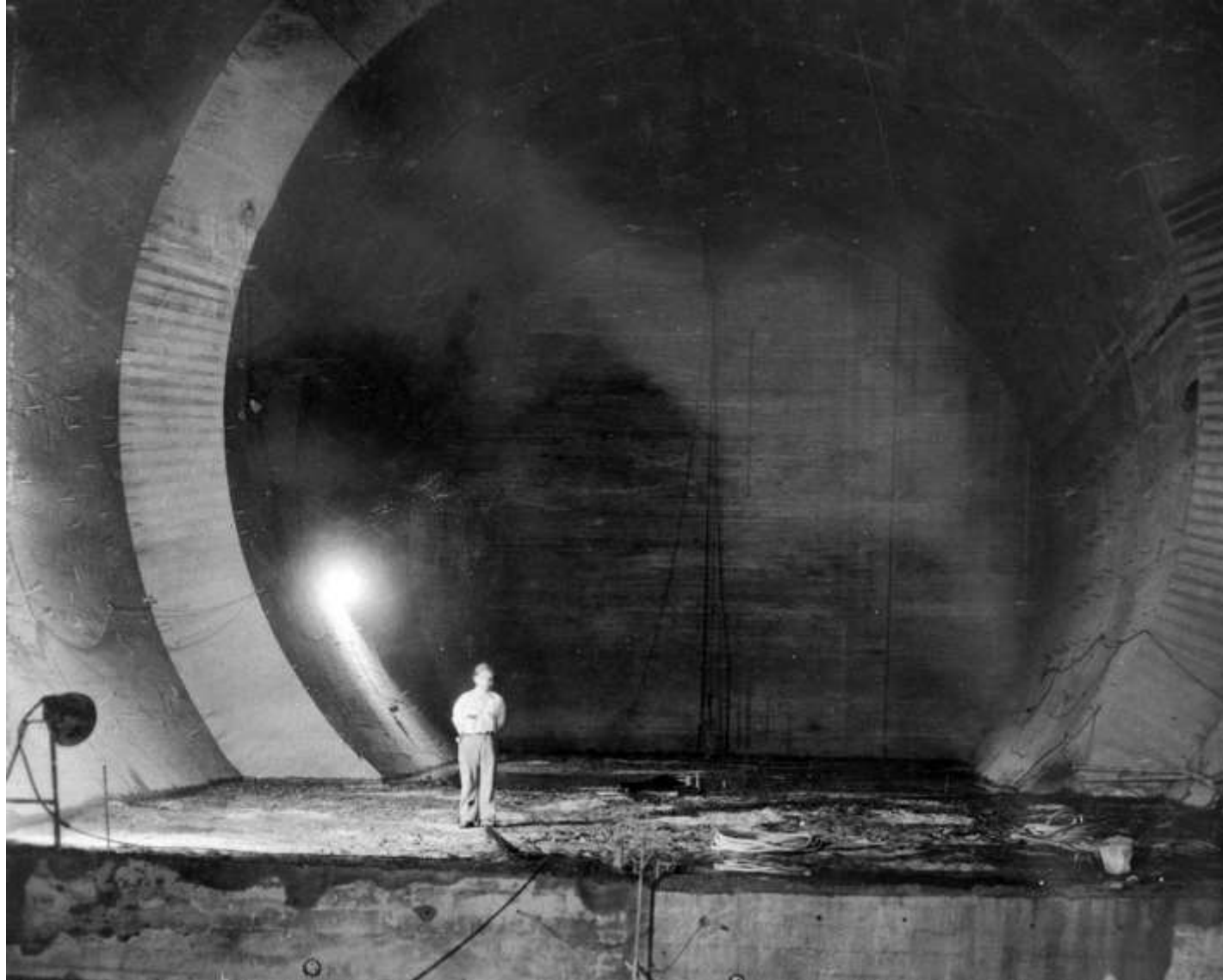
Upstream tunnel plug construction in Diversion Tunnel No. 3. This view shows the downstream face of the completed section of the plug with the lower pours of the next lift in place (June 1934)
