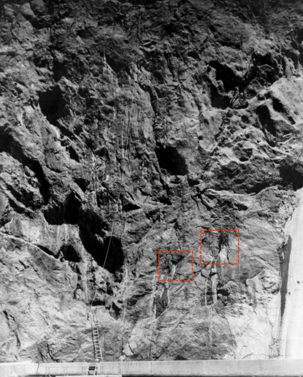
Seepage on the Nevada canyon wall (above roof of the central section of the Powerhouse; July 1938)
