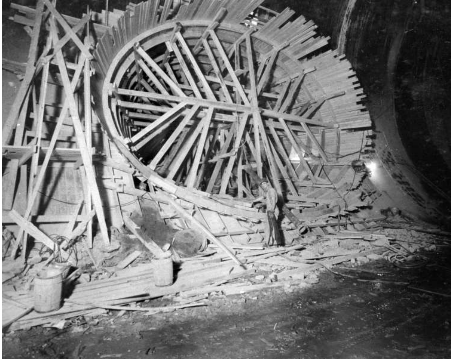
Timber formwork for intersection transition between Diversion Tunnel No. 3 and Penstock tunnel (June 1934)
