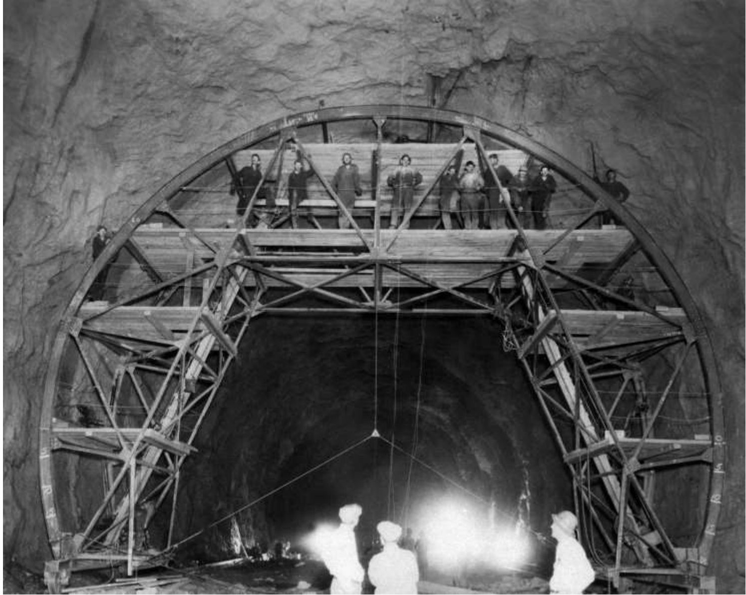
Close-up showing details of Trimming Jumbo used in scaling walls of diversion tunnels and removing projecting rock (April 1932)
