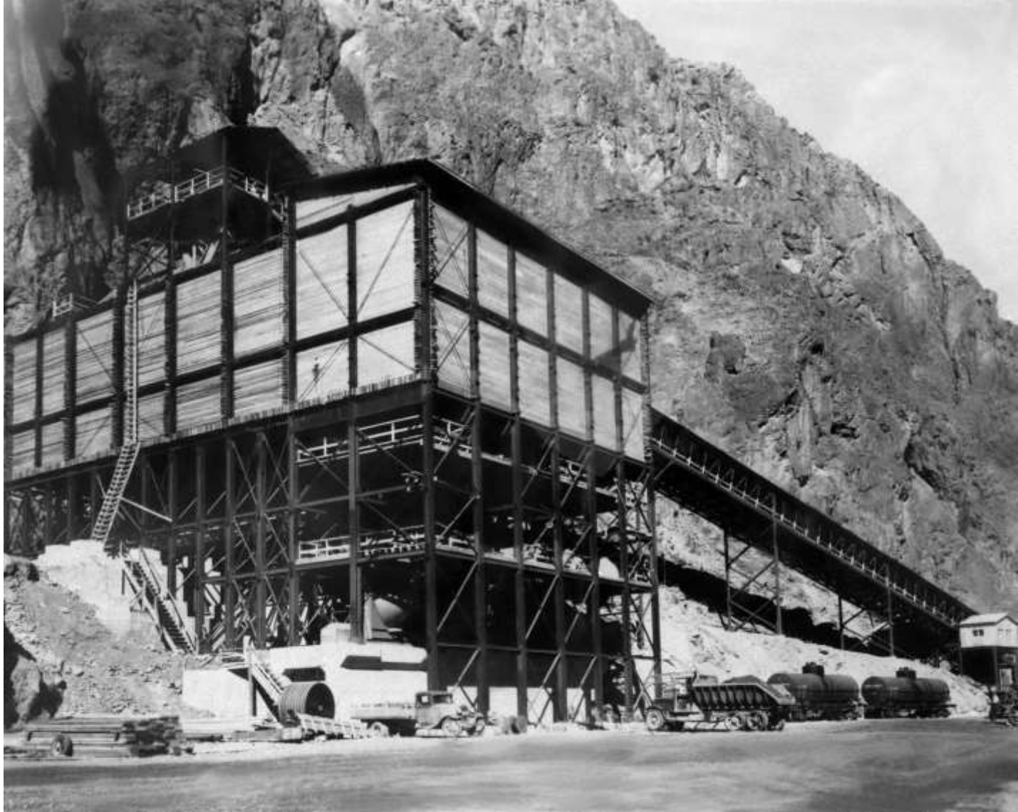
The Low-Level concrete mixing plant nearing completion. Silos for the storage of cement and bunkers for gravel storage were installed in the upper stories (January 1932).
