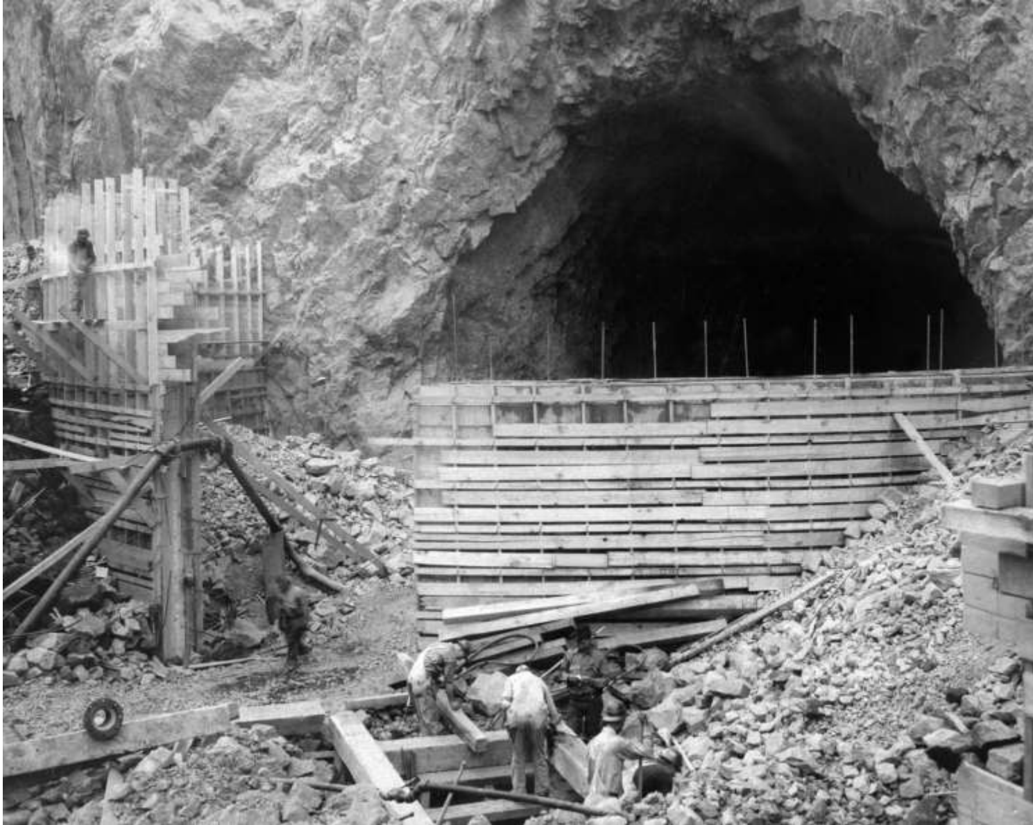
Semi-circular (arch) concrete Cofferdams being erected around the portal of Diversion Tunnel (as protection against high water; April 1932)
