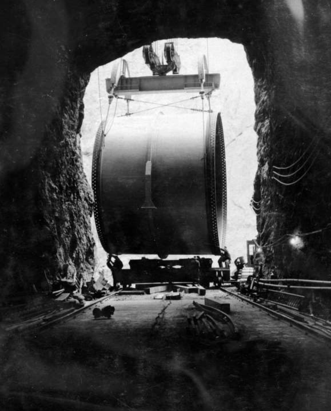
30-foot diameter penstock pipe section being lowered by cableway crane onto car at entrance to Penstock header tunnel (December 1934).
