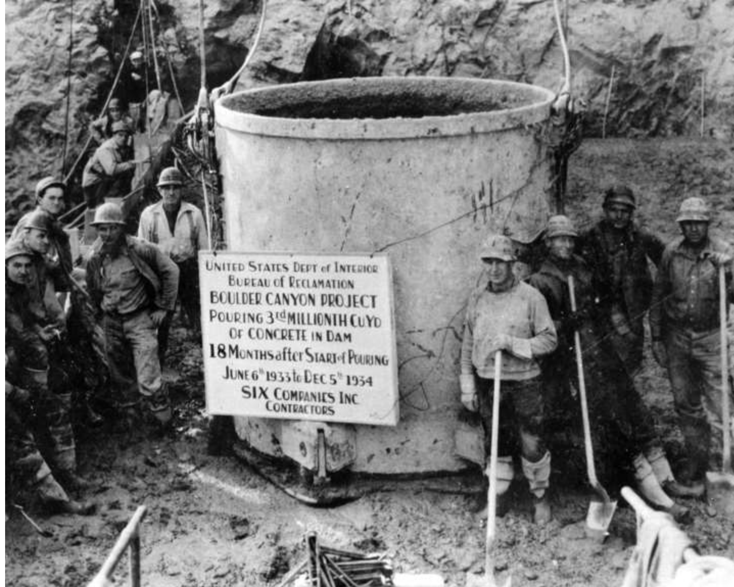
Placing the “third-millionth” cubic yard of concrete in Hoover Dam; December 5 th 1934
