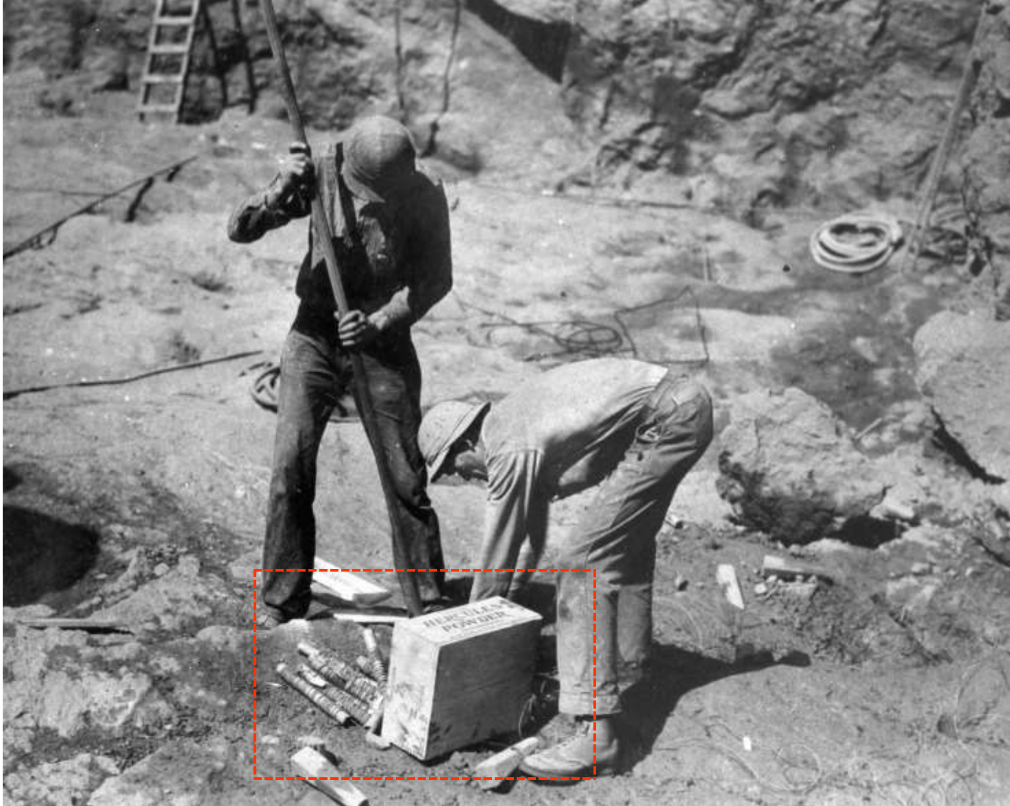
Workmen loading hole with dynamite preparatory to blasting (in the Nevada power plant site; March 1934)
