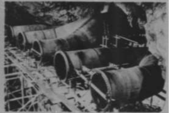
Outer conduit at No. 2 Plug
