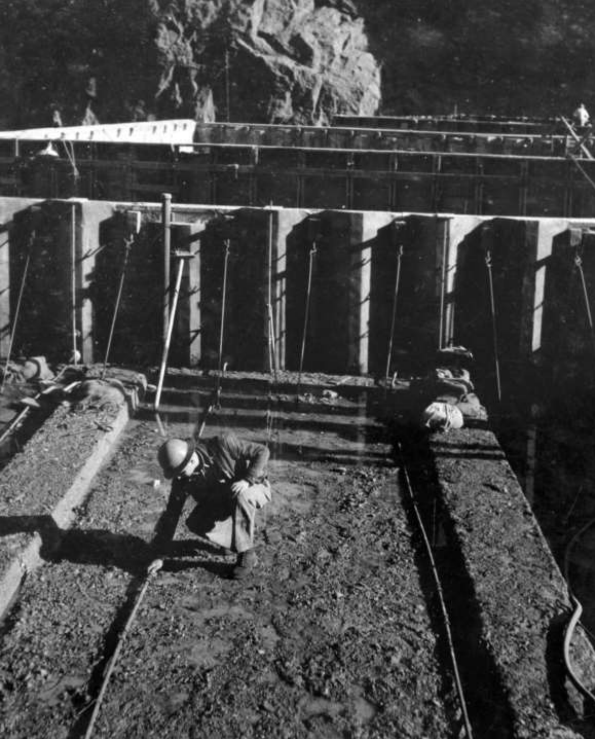
Photo showing the manner in which pre-cooling distribution pipes were installed on top of the concrete pour (March 1934)
