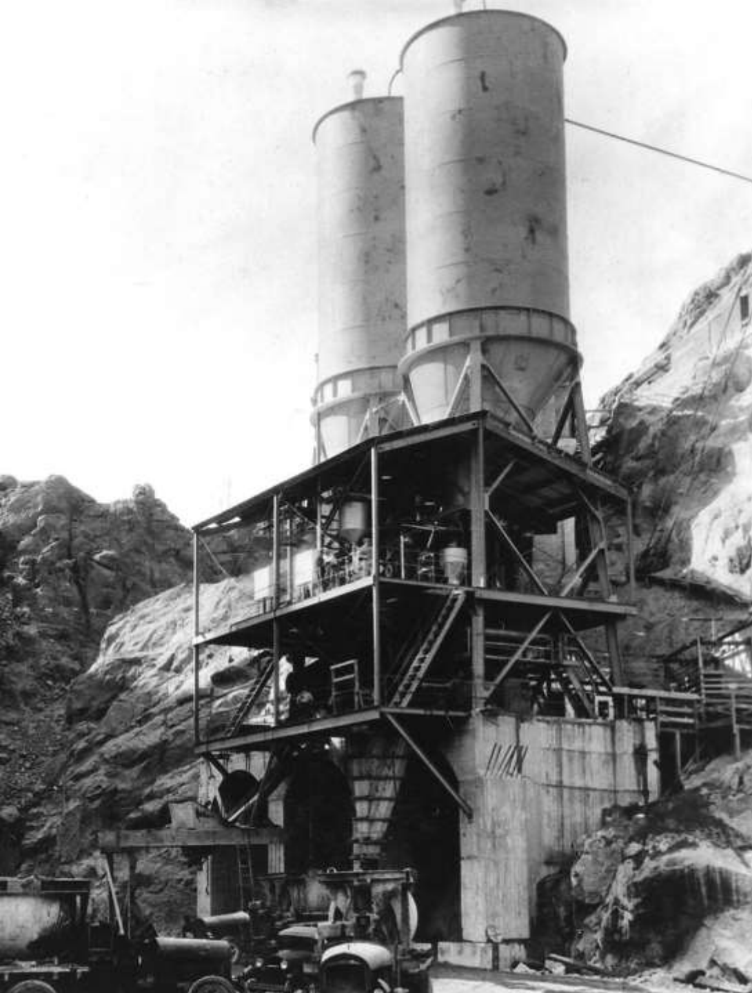
Six Companies' high level concrete mixing plant showing loading, mixing and control decks with cement storage silos above (March 1933)
