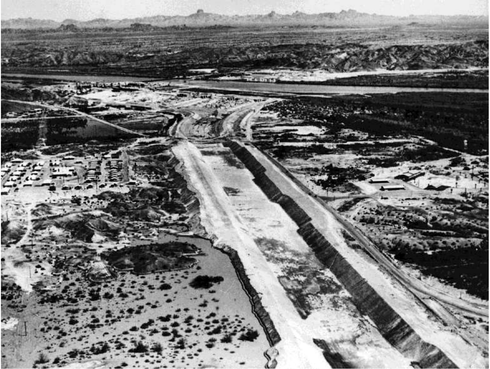
Looking upstream along the All-American Canal (from near Station 85 during construction; March 1937)
