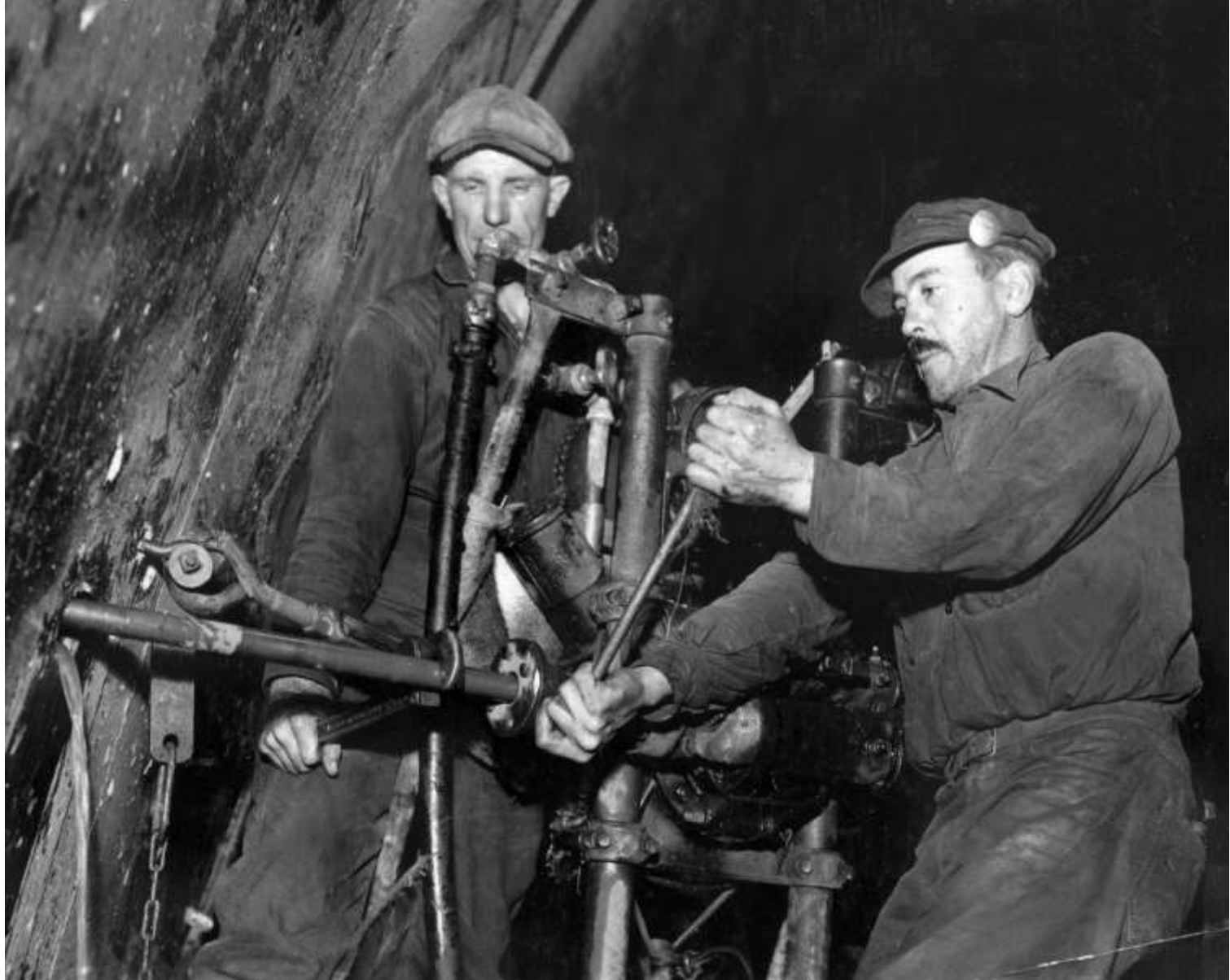
Driller tightening the chuck after pulling the chuck back in order to drill another three-feet (December 1940).
