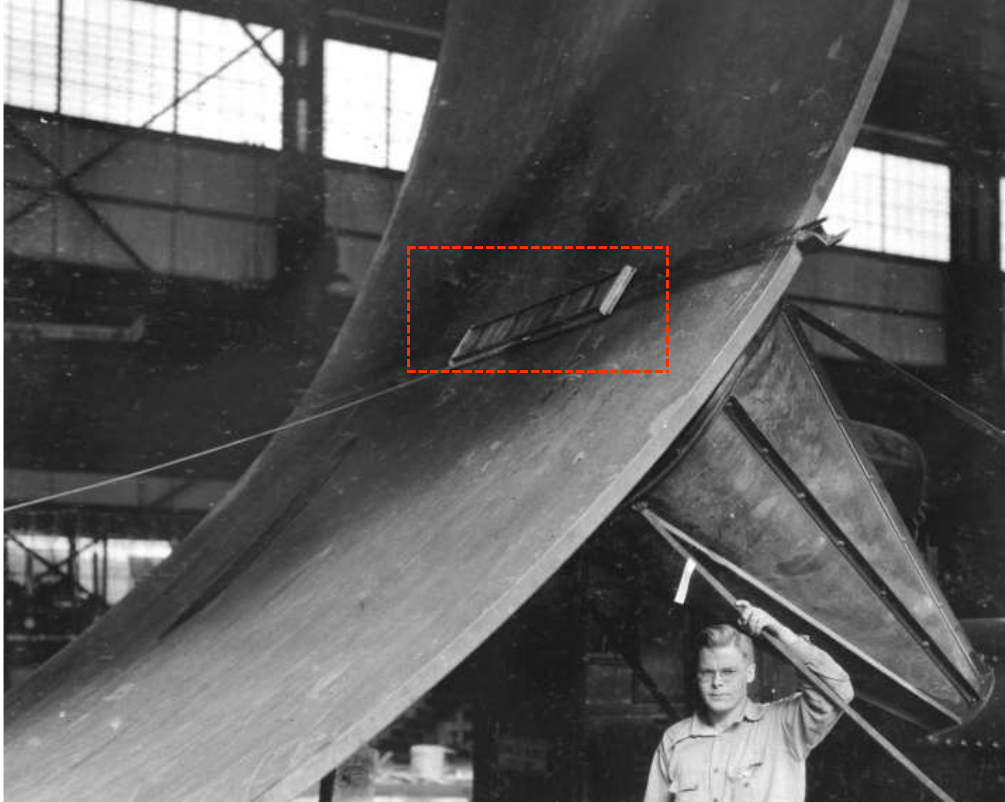
X-ray machine set up on thirty-foot diameter pipe section for exploration of longitudinal welded seam (note film holder supported inside pipe; October 1933)
