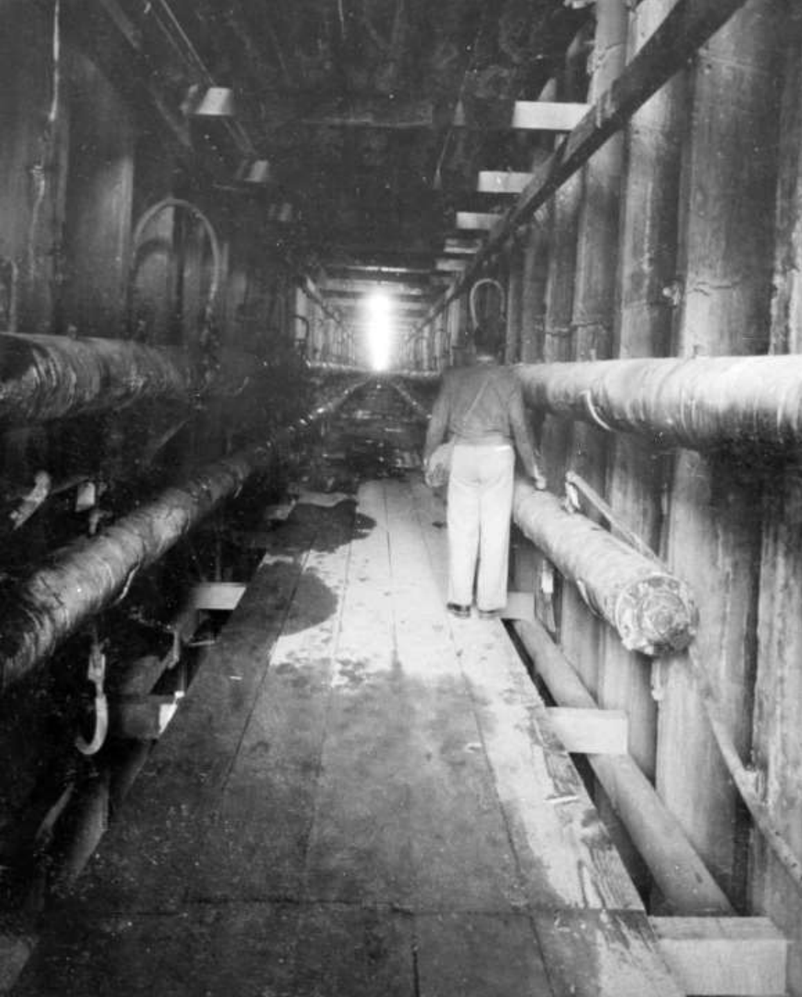
Cooling system header pipes in eight-foot wide slot through middle radius of dam structure. View looks downstream through slot at Elevation 680 (November 1933).
