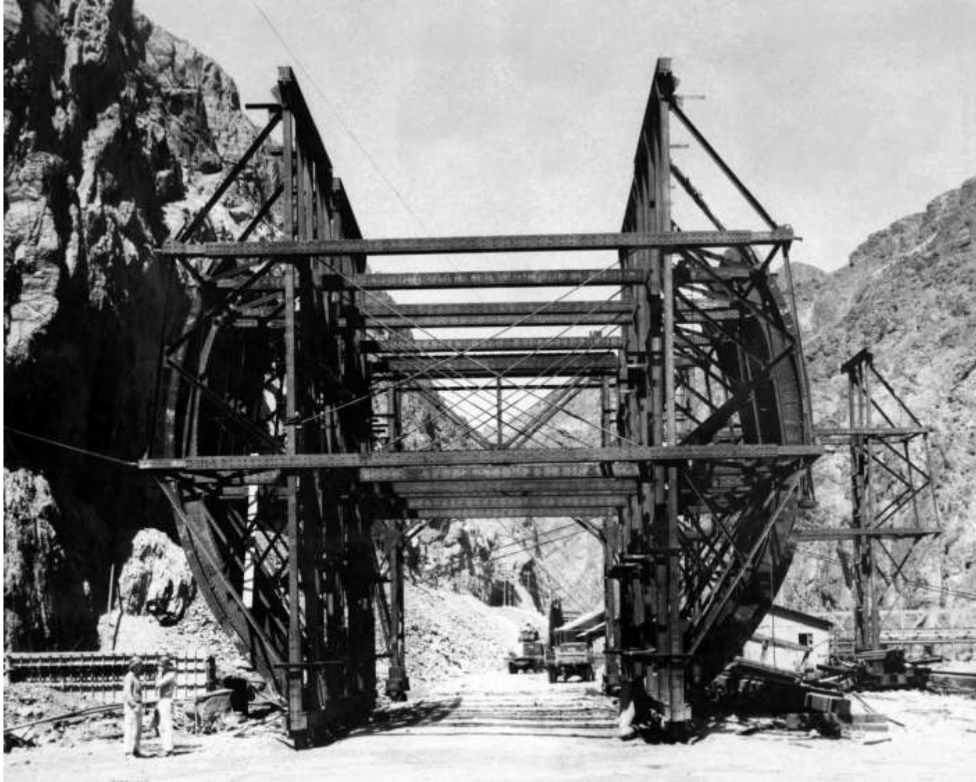
Fabricated steel forms for placing the three-foot thick lining in the side-wall section of the Diversion Tunnels being erected outside the upper portal of Diversion Tunnel No. 1 (July 1932)
