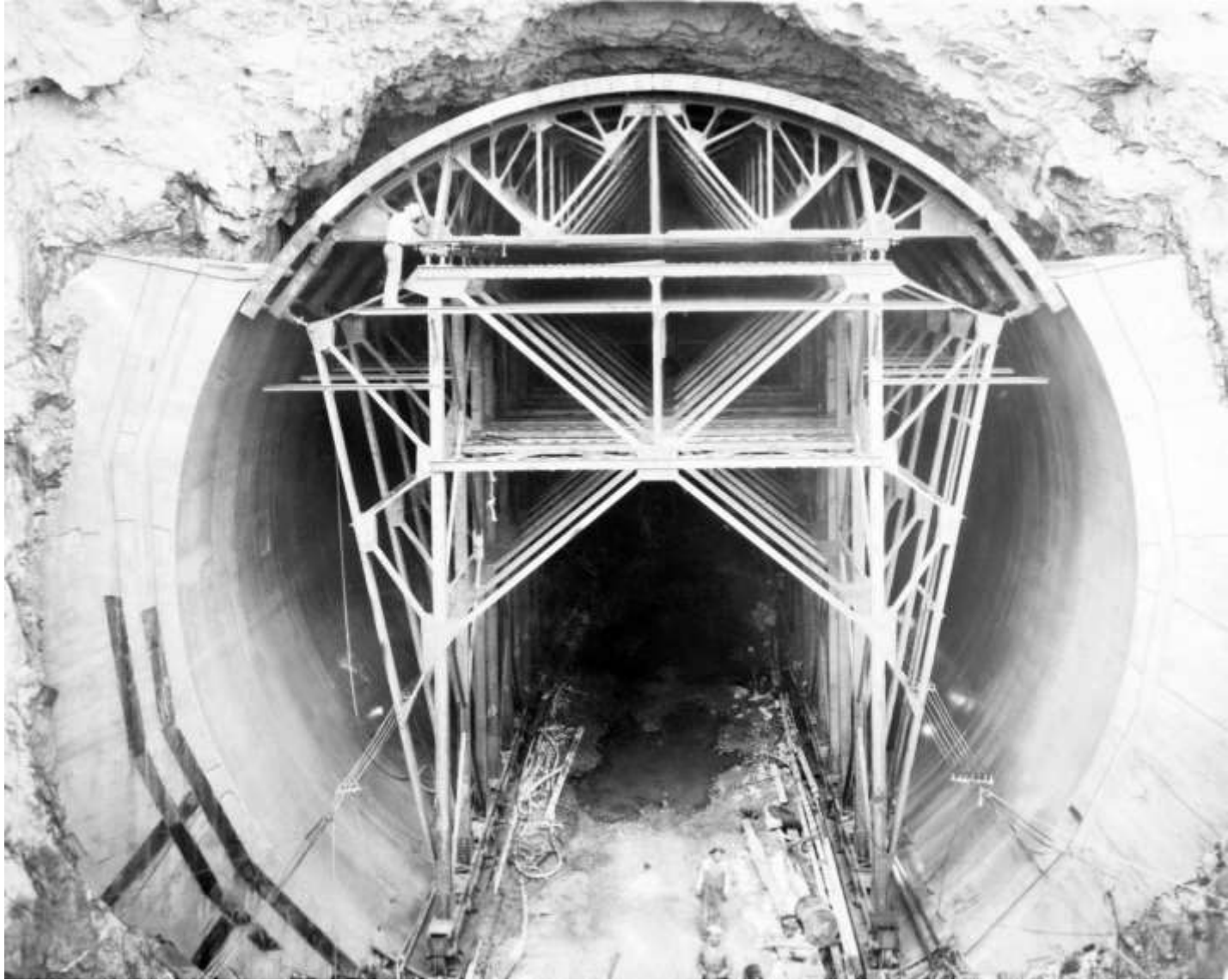
Placing steel form for the first pouring of concrete in the lining of the arch section of the Diversion Tunnels. View shows upper portal of Diversion Tunnel No. 4 (June 1932).
