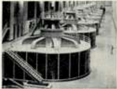
Nevada wing of power plant
