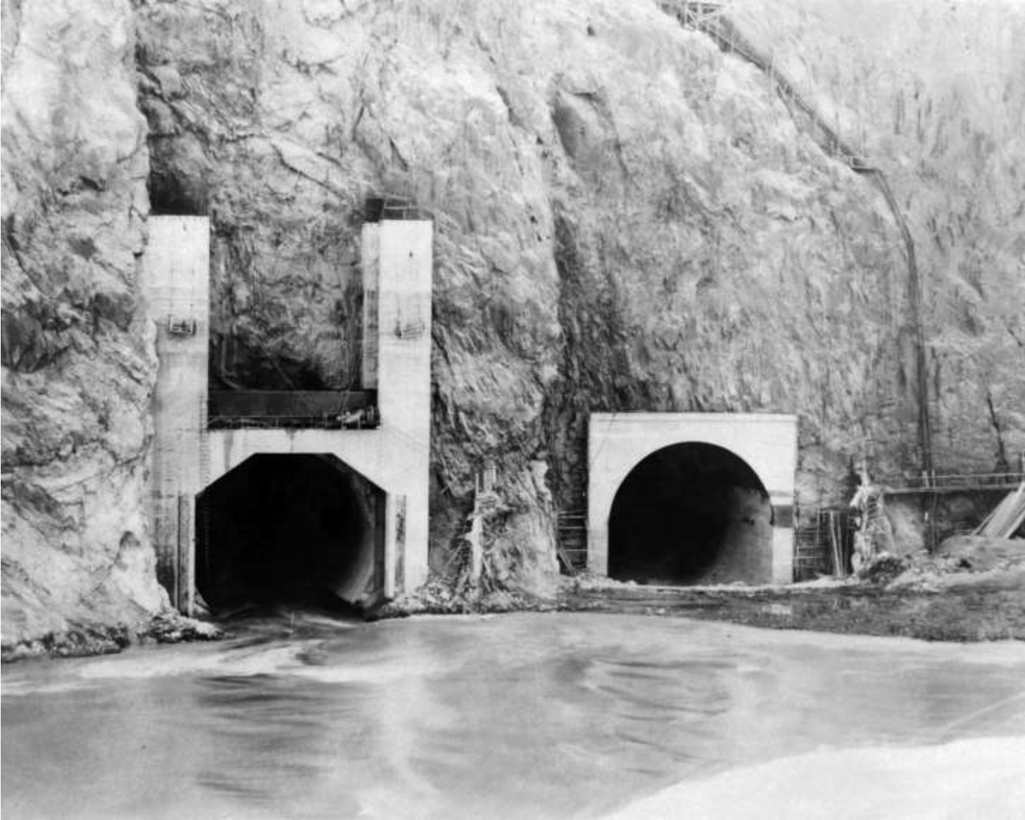
Close-up of upper portals of Diversion Tunnels Nos. 3 (inner) and 4 (outer) showing flow in Diversion Tunnel No. 4 (at left, shortly after blast; November 13th 1932)
