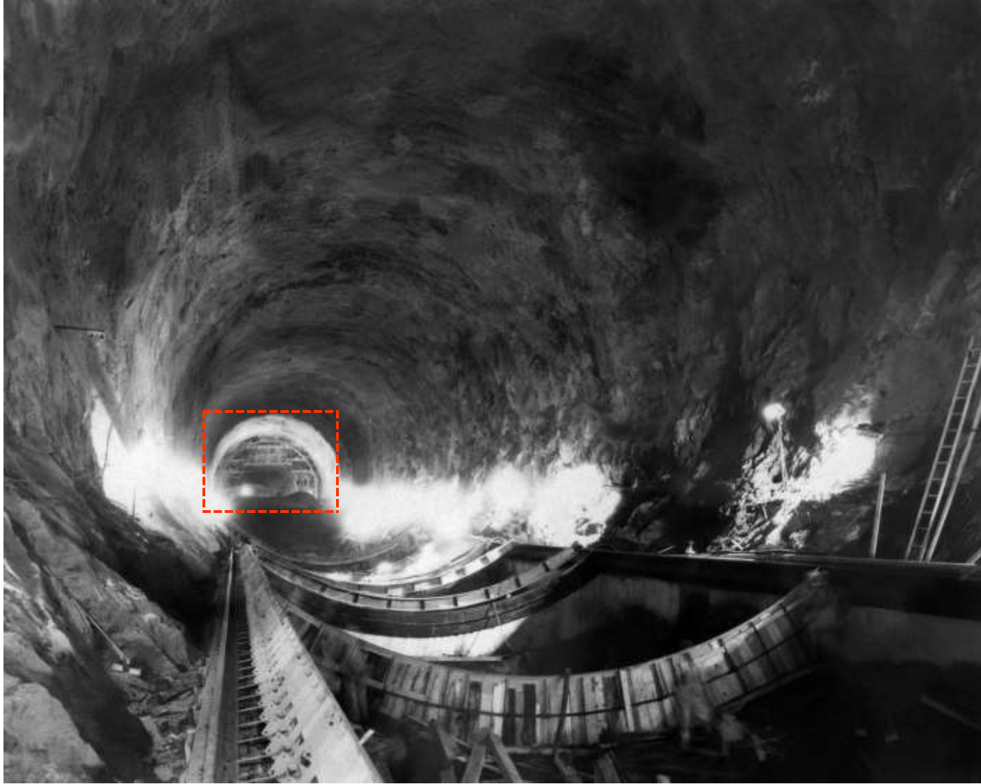
Invert forms in upper Diversion Tunnel No. 3 (showing method of pouring slabs). Trimming Jumbo (for aligning gauge of tunnels) in background (March 1932).
