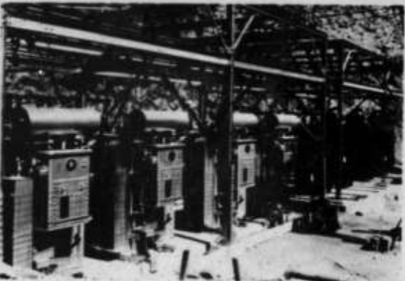
BOULDER CITY AND LAS VEGAS SUBSTATIONS
