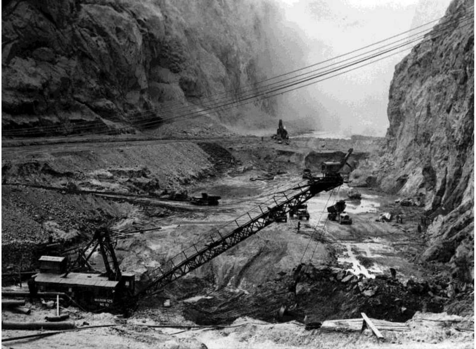
Looking downstream into the Upper Cofferdam excavation (dyke and restricted river channel are at left; October 1932)
