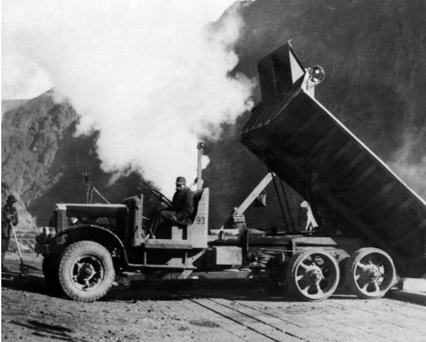
A ten cubic yard Moreland truck dumping directly in the side-dump railroad cars at the dump hopper (in front of the low level mixing plant). Truck was carrying muck from upper portals of the Diversion Tunnels (January 1932).
