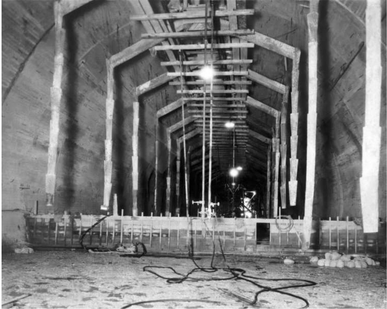
View taken from the upstream end of No. 4 Plug, looking downstream (showing method of pouring; April 1935)
