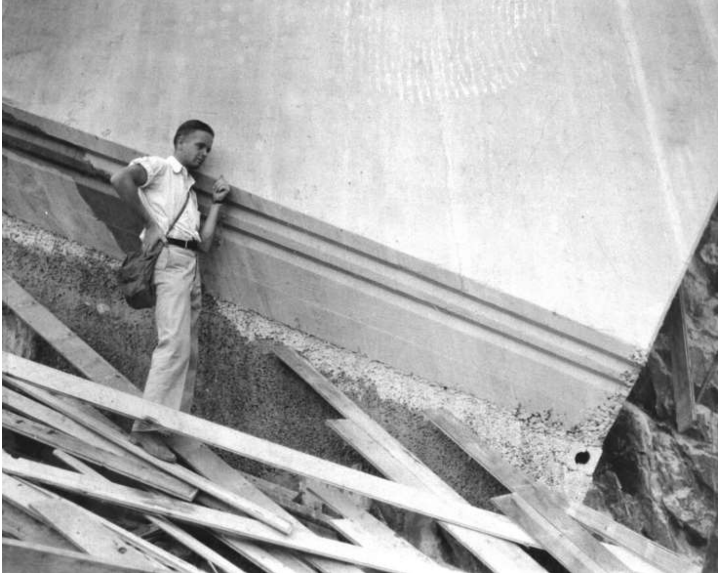
Construction joint (at base of side-wall) along vertical curve transition into inclined Spillway tunnel (Nevada Spillway; September 1933)
