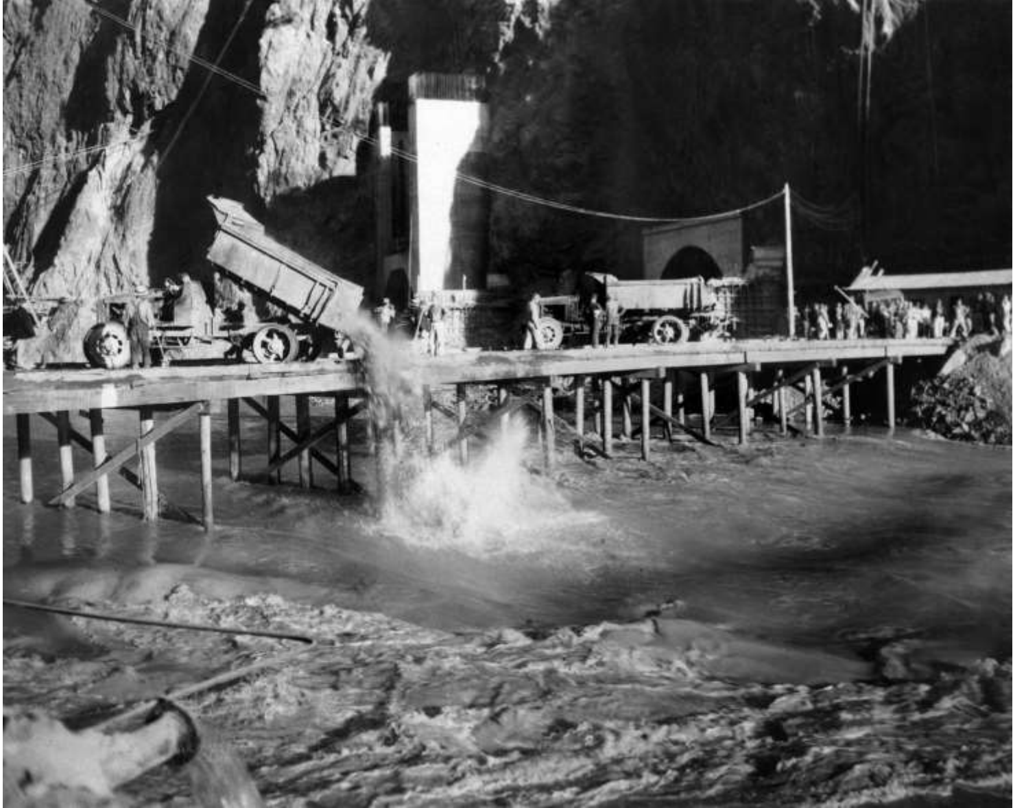
Dumping materials at temporary pile (trestle) bridge to complete diversion of the Colorado River (after blast; November 13 th 1932)
