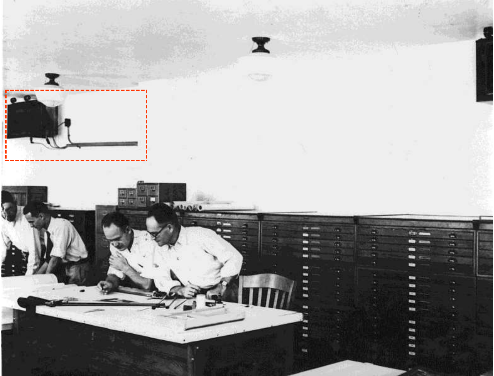
Cooling units installed in the office engineer's drafting room at the Government Administration Building, Boulder City
