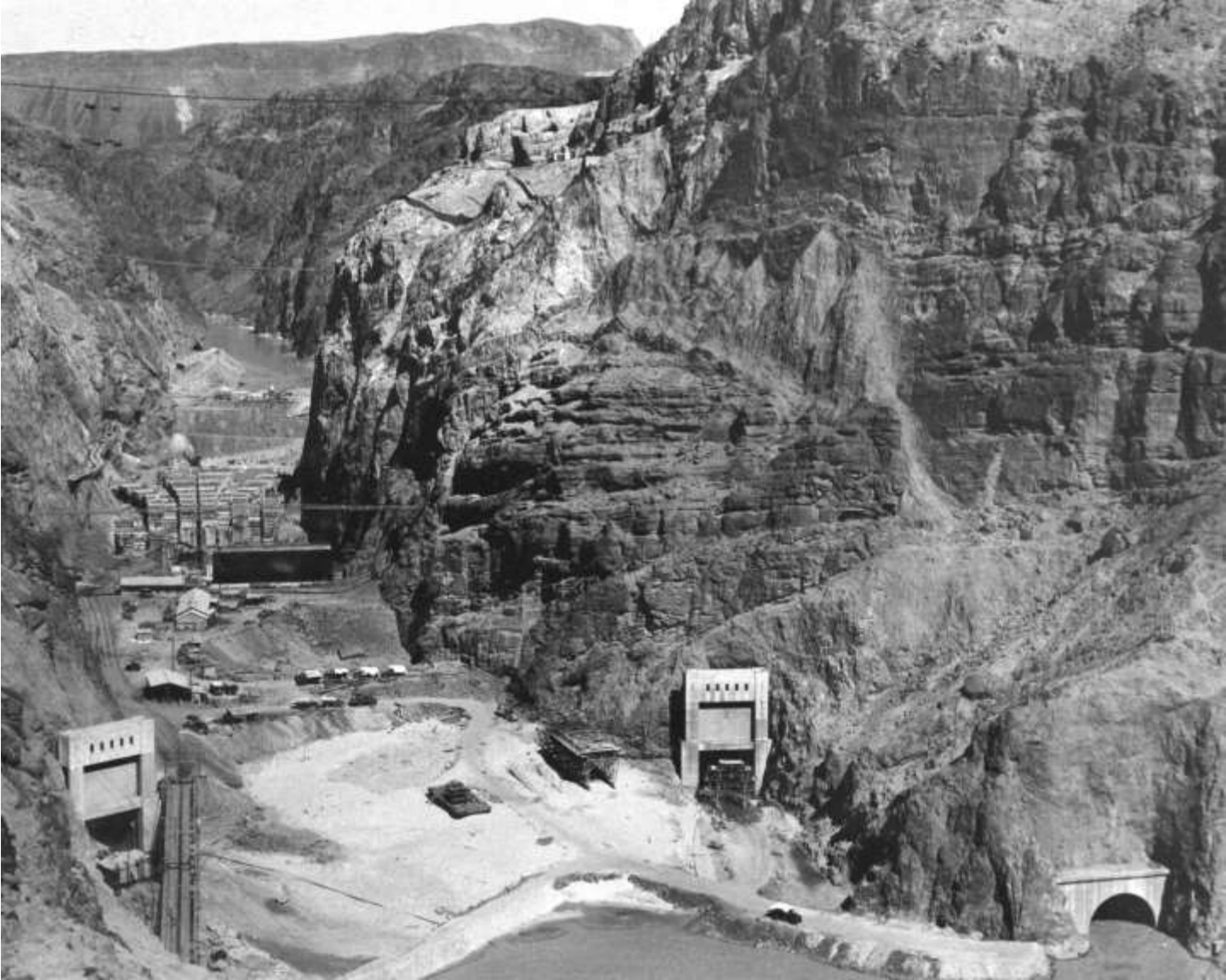
Looking upstream through Black Canyon (from permanent camera station). View shows dam structure and outlet portals of diversion tunnels Nos. 2, 3 and 4 (September 1933).
