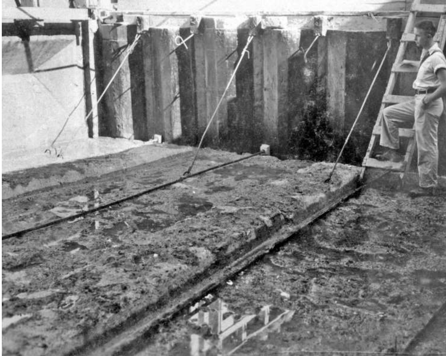
Cooling system pipes installed on top of five-foot pour (note horizontal construction joint-key construction joint-key; October 1933)
