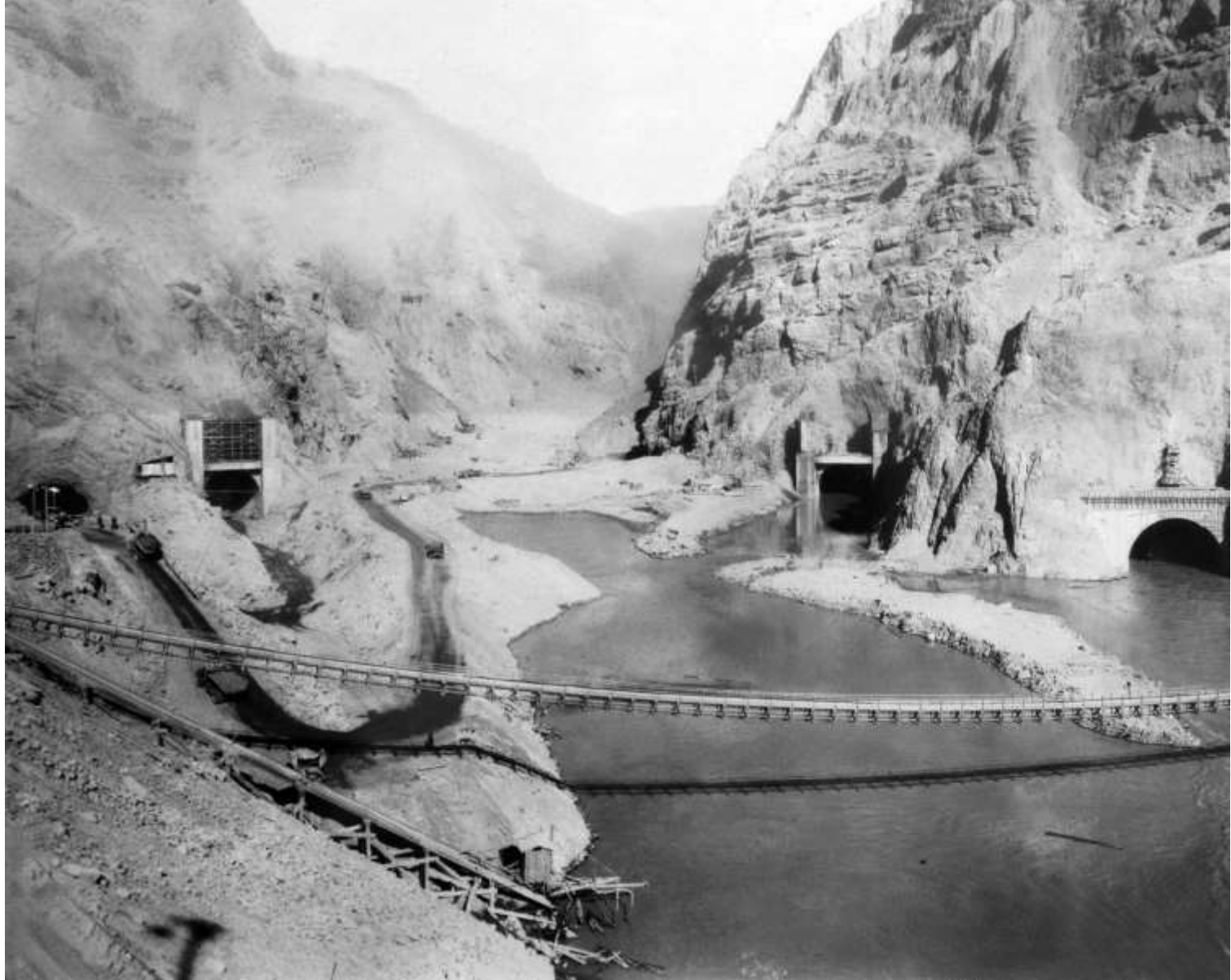
Lower Portals of the Diversion Tunnels and excavation in the river bottom (for Downstream Cofferdam and rock barrier; January 1933)
