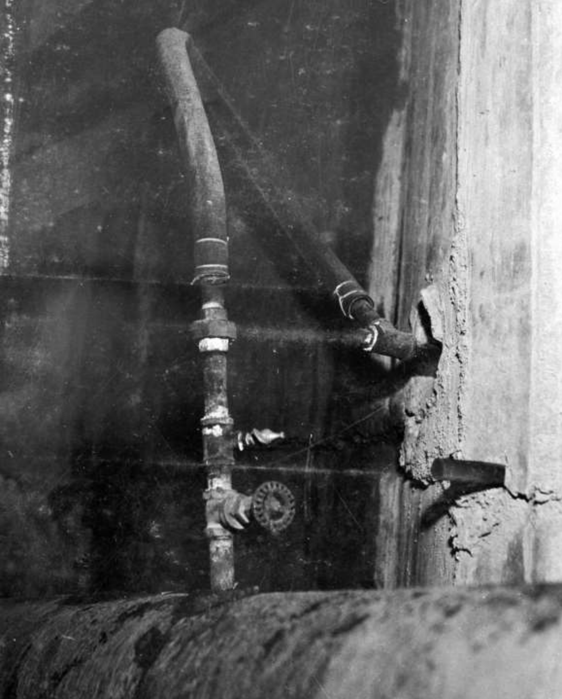
Detail showing connection from header pipe to circulating system in the dam's pre-cooling system (February 1934)
