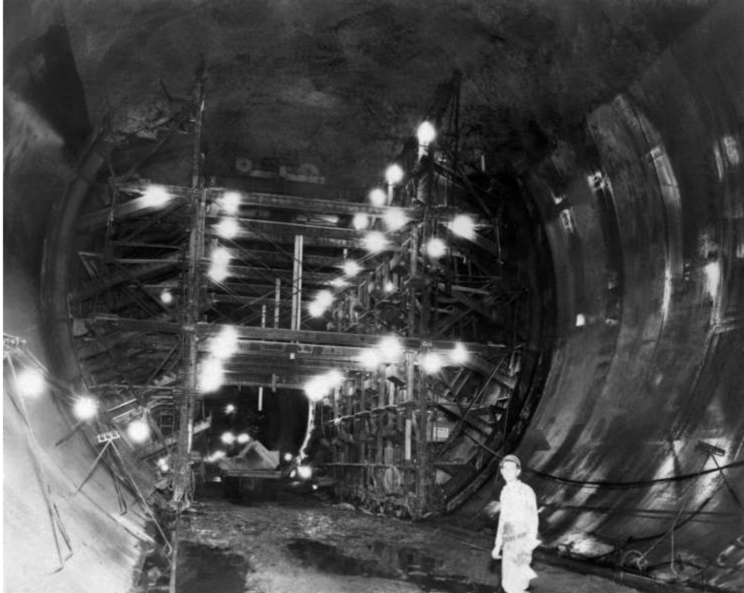
Showing the method of construction and operations of the Side-Wall Jumbo for placing the lining in the Diversion Tunnels (June 1932)
