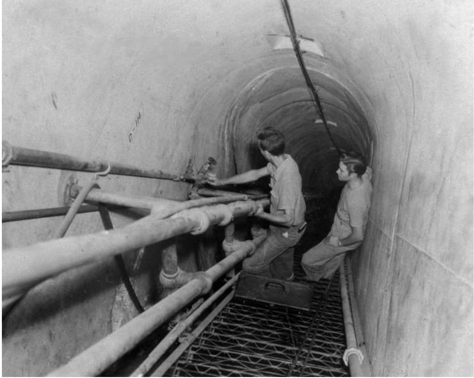
The grout was pumped through pipes through the Inspection Galleries deep into the dam (October 1940)
