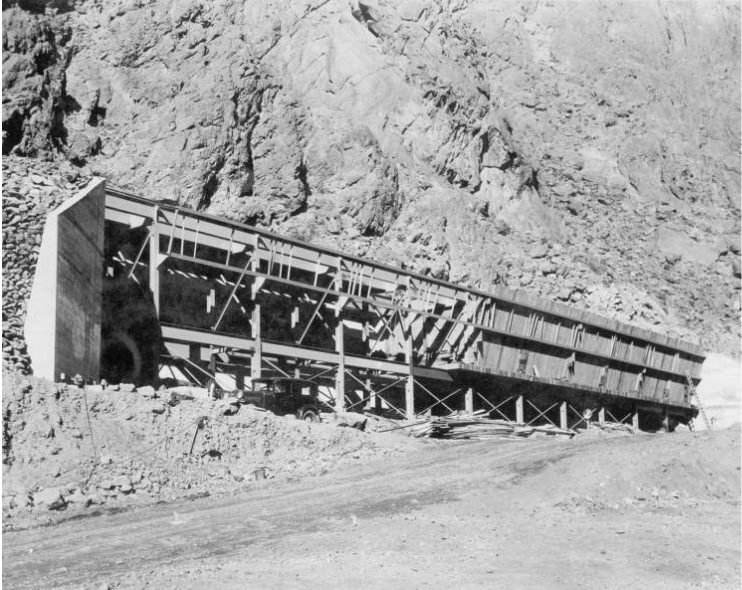
Aggregate bins at Six Companies' Low-Level concrete mixing plant. Conveyor to mixing plant operates from end (at left; Dec. 1931)
