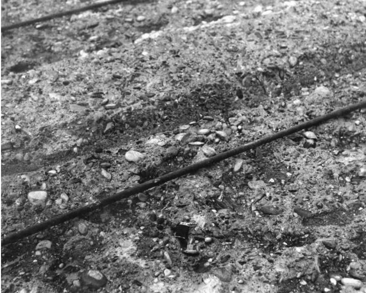
Detail of construction joint cleanup showing cooling system pipes and horizontal construction joint keys (test pour in Column H-5, Elevation 630; August 1933)
