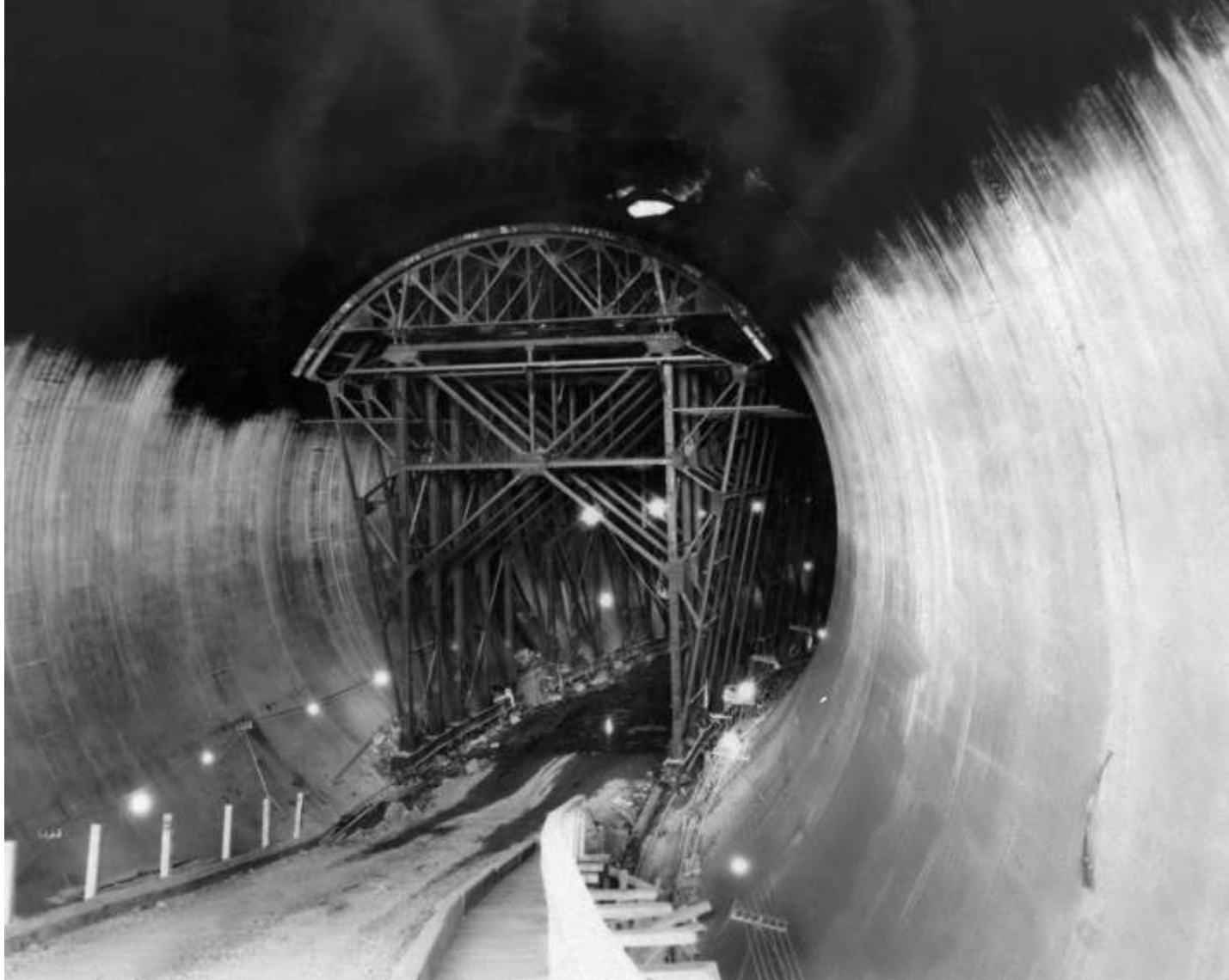
Interior of Diversion Tunnel No. 4 (near the upper portal) showing the Arch Jumbo in place. The arch section has been coated with a bituminous surface for curing the concrete (June 1932).
