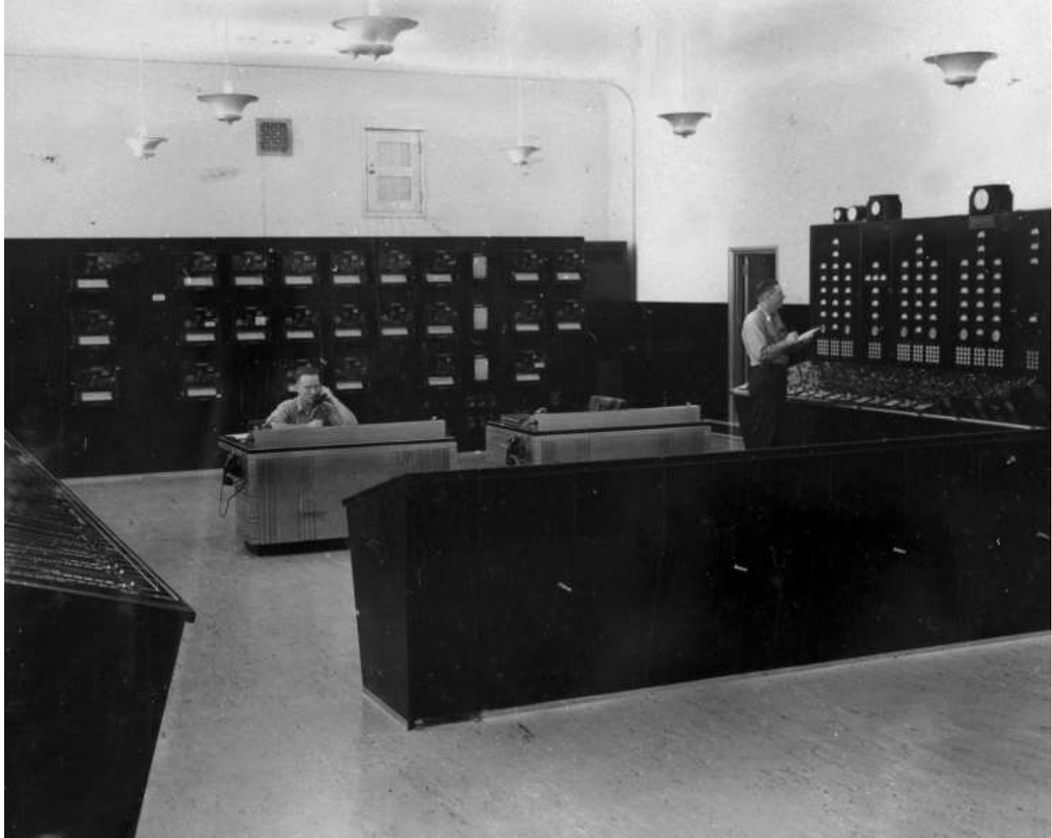
General view of the Main Control Room located in the central section of the Powerhouse (November 1939)
