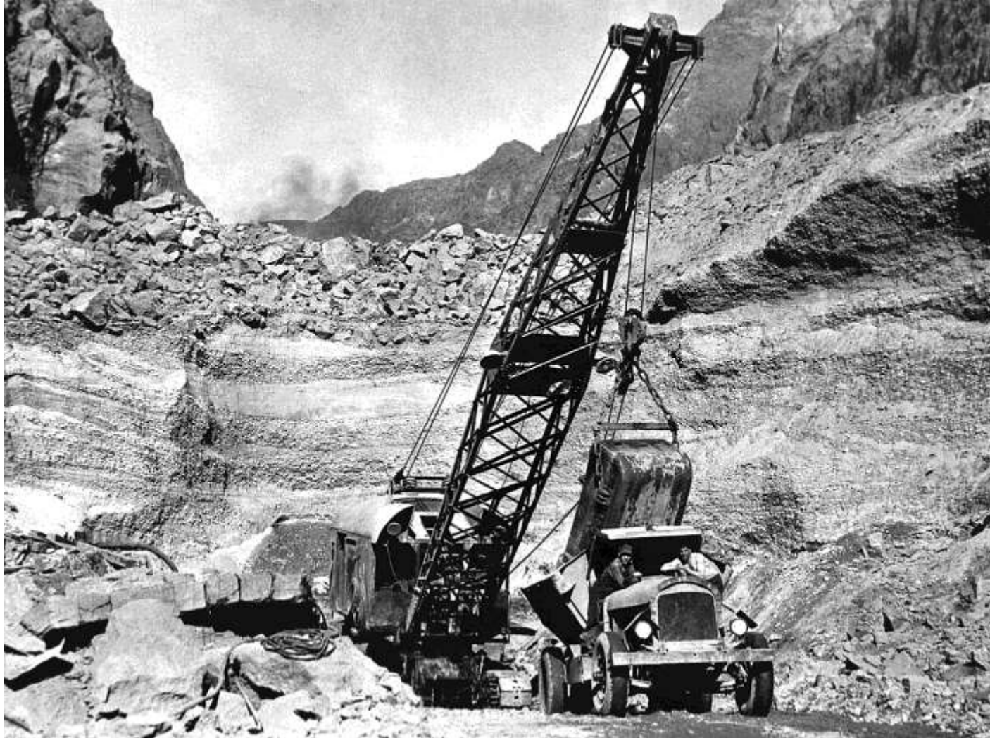
Looking upstream through Black Canyon toward the dam site (showing condition after the diversion of the Colorado River). Lower levels of canyon choked with material blasted and scaled from the canyon walls. A downstream rock barrier can be seen in foreground (January 1933). 504
