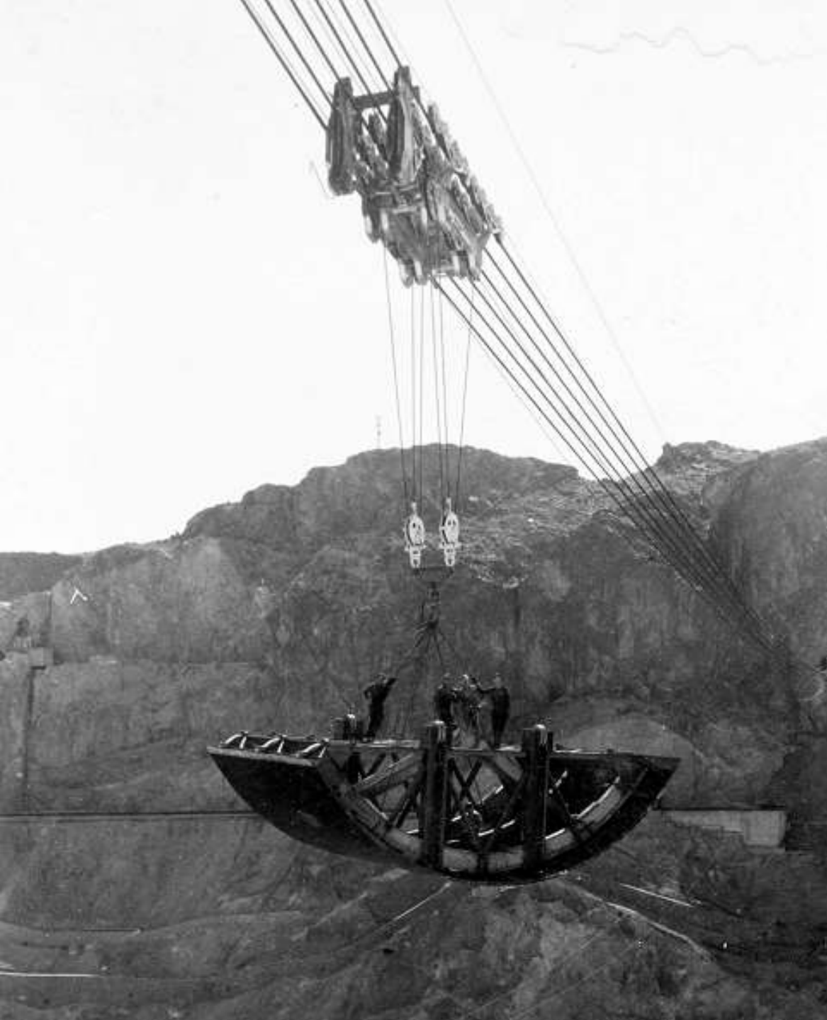
The 150-ton cableway transporting Penstock header tunnel lining forms into canyon (September 1933)
