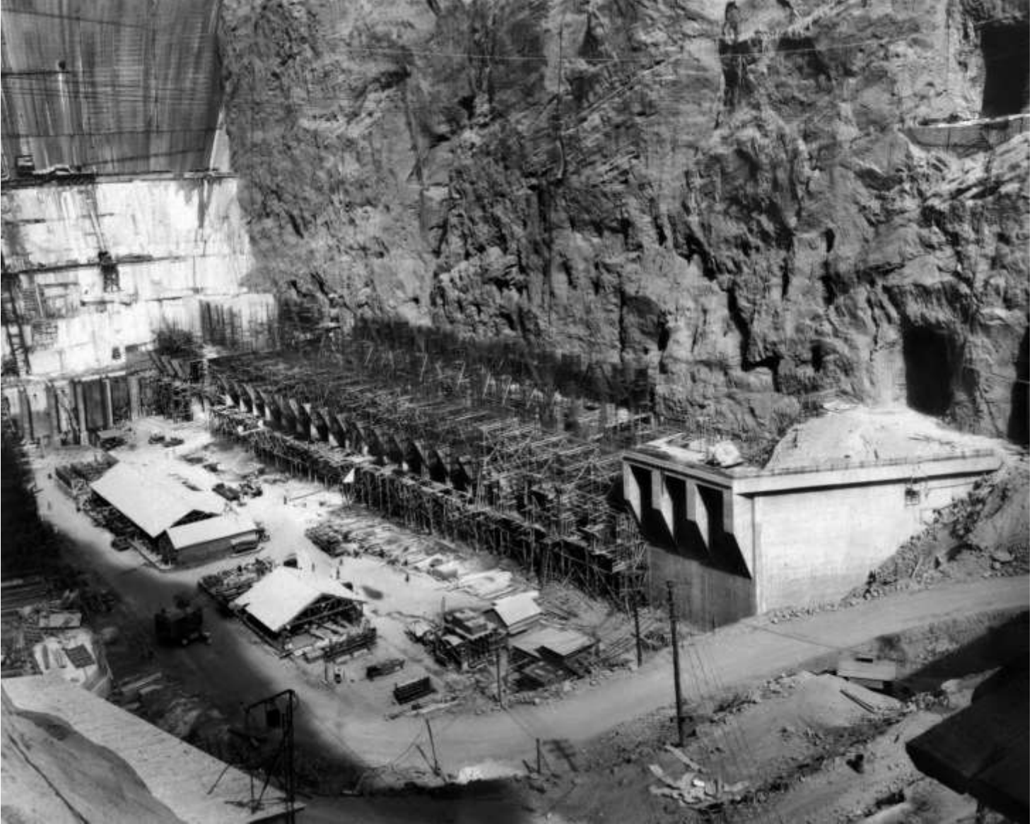
Arizona Powerhouse (from the Nevada Valve House Bench ; August 1934)
