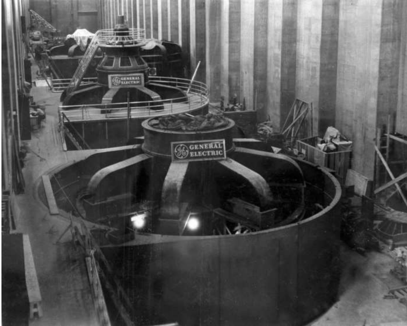
The four 82,500 Kva generators of the initial power installation, in various stages of erection in the Nevada wing of the Powerhouse. Two were furnished by General Electric , two by Westinghouse (October 1936). 791
