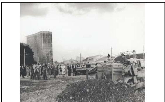
The first sod is turned on the Construction Site of the SOH (March 2 nd 1959) 293
