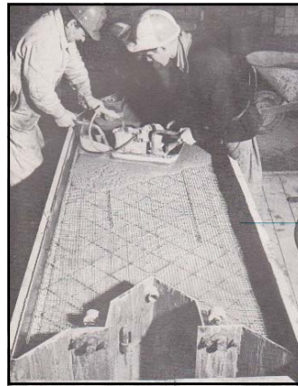
Pouring grout over the reinforcing mesh and back-surface of tiles in chevron-shaped Tile Lid
