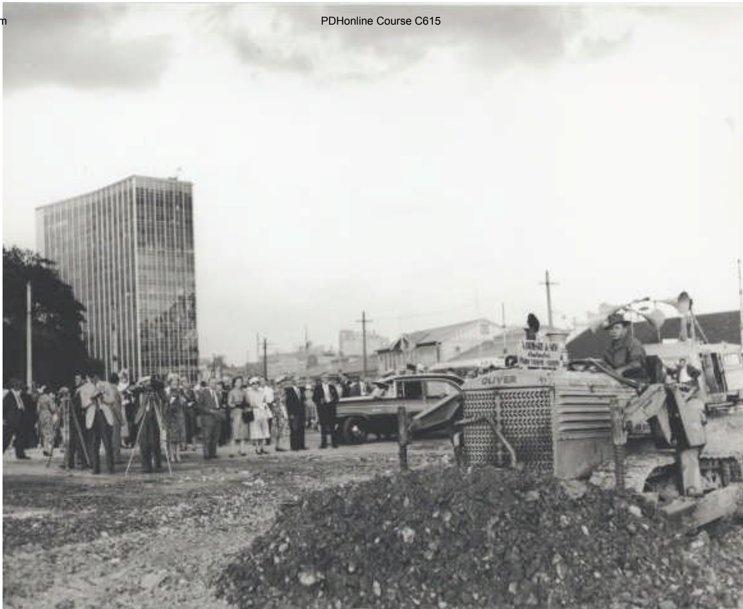
The first sod is turned on the Construction Site of the SOH (March 2 nd 1959)
