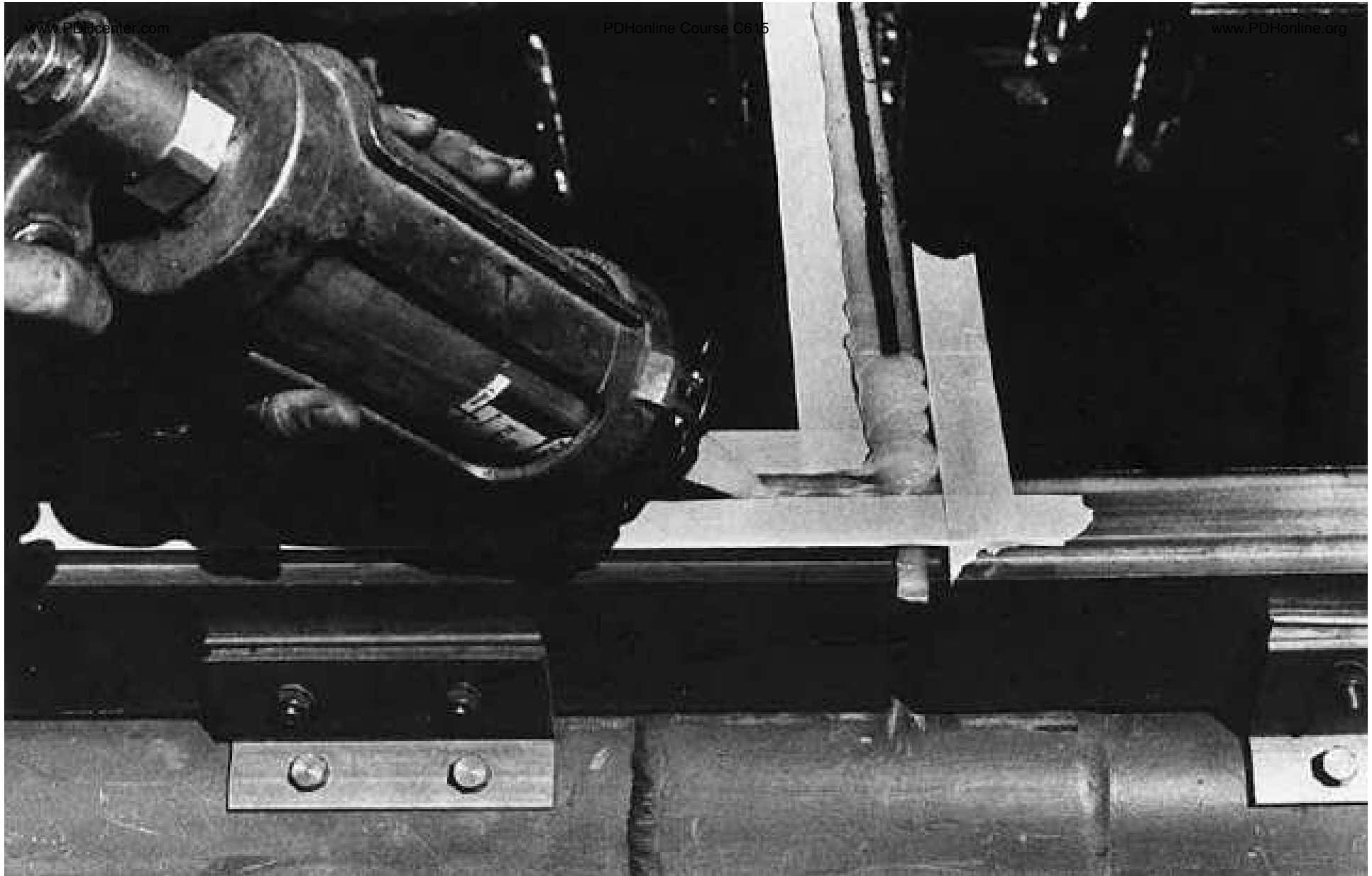
Silicone sealant being applied to the extruded bronze T-joint prior to installation of the glazing bar
