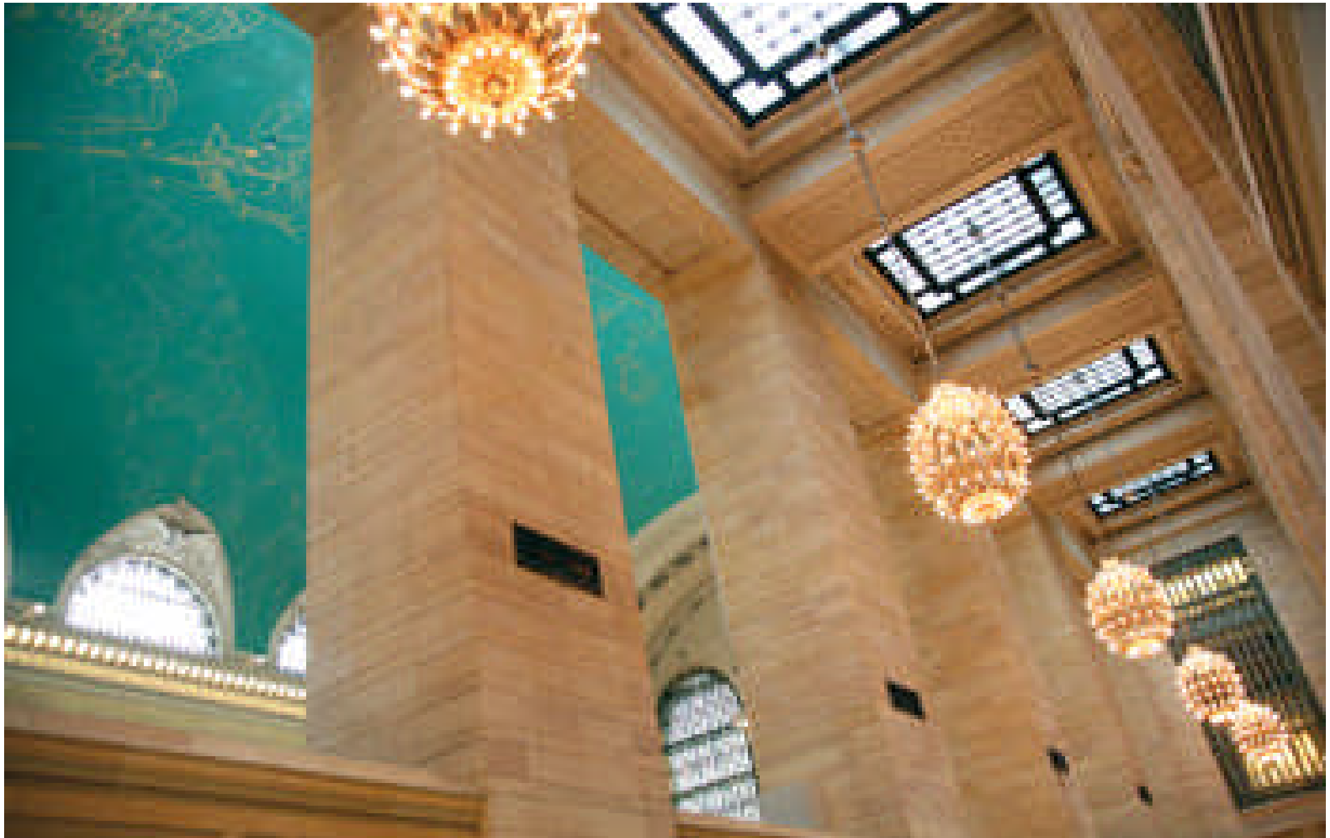
Above: interior view of four of the twenty-four foot square roof skylights that were restored as part of the roof repair work
