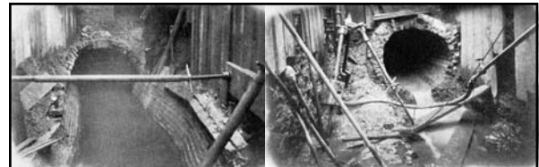
"...There were some special problems to be solved at certain points. The road crossed one or two sewers in places where, owing to the low elevation of the ground, it was not possible to carry them down beneath the railway bed. At Canal Street there was a sewer nine feet wide and six feet high, which drained an area of one hundred and twenty one acres lying east of the road, and ran across Broadway to the Hudson River. In this case a new channel, six feet in diameter, was built from the East River up James, Mulberry, and Center Streets to Canal Street, so that now the drainage of that district will be conveyed eastward instead of to the west..." John B. McDonald, 1902 Left: Bleeker Street sewer Right: 157th Street sewer
