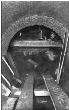
A notable example of sewer diversion was at Canal Street where the flow of the sewer was carried into the East River instead of the Hudson River permitting the sewer to be bulk-headed on the west-side and continued in use. On the east-side a new main sewer was constructed to empty into the East River. The new east-side sewer was built off the route of the Subway for over a mile. An interesting feature in the construction was the work at Chatham Square, where a 6.5-foot circular brick conduit was built. The confluence at this point of numerous electric car lines, elevated railroad pillars and voluminous vehicular street traffic made it imperative that the surface of the street not be disturbed thus the sewer was built by tunneling. This tunneling was through very fine running sand and the section to be excavated was small. To meet these conditions, a novel method of construction was used. Interlocked "poling boards" were employed to support the roof and were driven by lever jacks (similar in manner to the method used in the shield system of tunneling). The forward ends of the poling boards were supported by a cantilever beam. The sides and front of the excavation were supported by lagging boards laid flat against and over strips of canvas which were rolled down as the excavation progressed. The sewer was completed and lined in lengths of from one-foot to 4.5-feet and at the maximum rate of work about twelve-feet of sewer were finished per week. Left: caption: "Special construction of 6.5-foot sewer, under Chatham Square"
