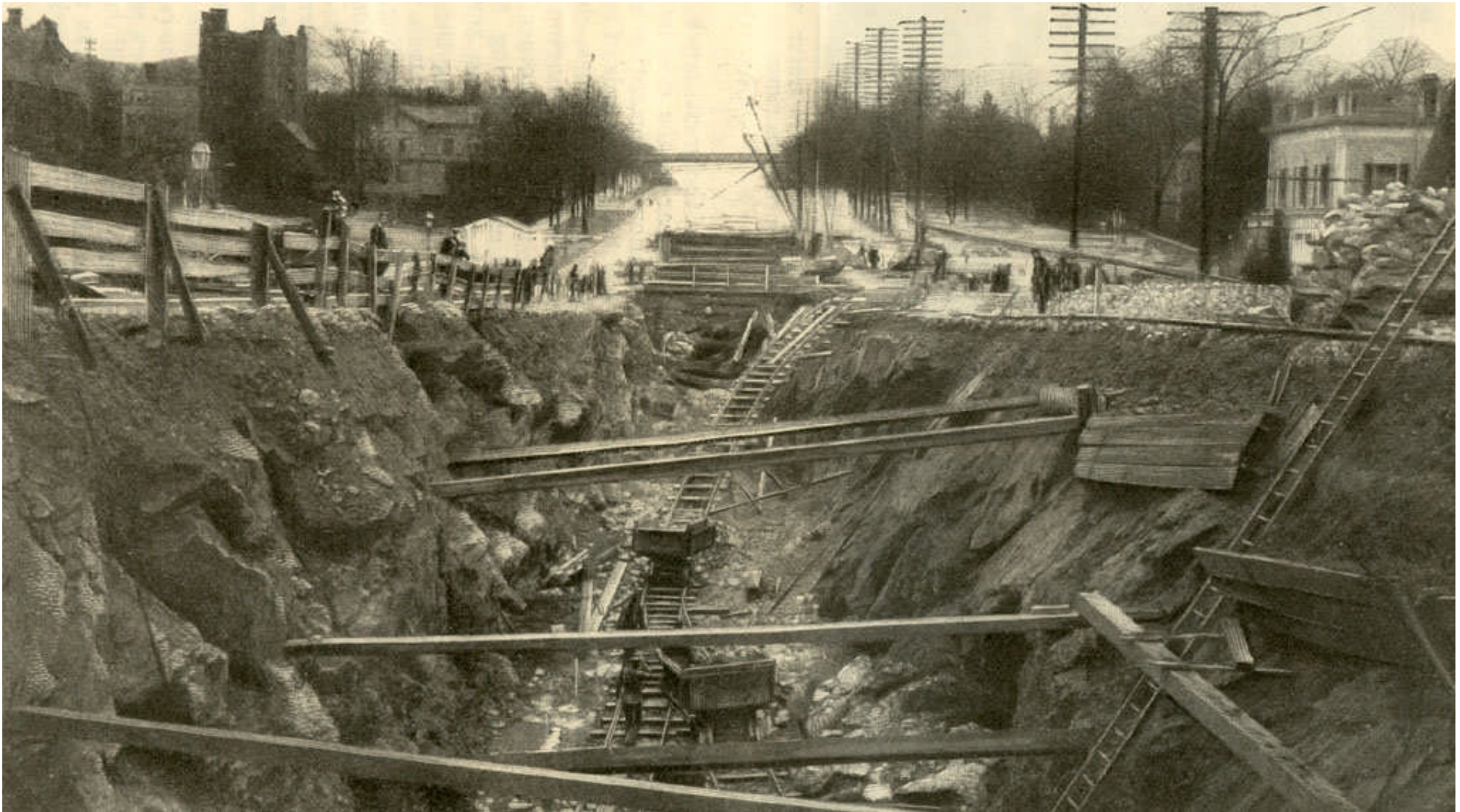
Above: caption: “View of the work on Broadway, looking south from One Hundred and Fifty Seventh Street, toward Trinity Church Cemetery. Both north and south of this point are hills through which a tunnel is being driven, the northern tunnel being nearly two miles long.”
