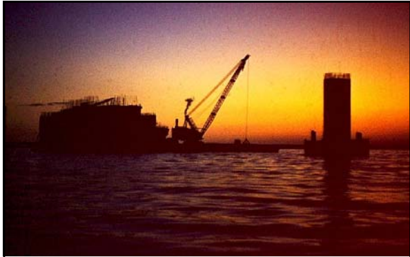
Above: caption: "Dredging barge and crane (the south anchorage is at left)." 163
