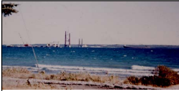
Above: caption: "This is in mid-summer 1955 and steel workers are assembling the two prefabricated main Mackinac Bridge towers."
