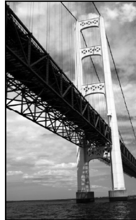
"...The main span at Mackinac is a suspension bridge, which is inherently the safest type of bridge. The stiffening trusses are 38 feet deep, or one-hundredth of the span length. This is 68 percent greater than the corresponding ratio of the Golden Gate Bridge. But even without this generously high depth-ratio, the Mackinac suspension span would have more than ample aerodynamic stability. In fact, by utilizing all of the new knowledge of suspension bridge aerodynamics, particularly my own mathematical and scientific discoveries and inventions, I have made the Mackinac Bridge the most stable suspension bridge, aerodynamically, that has ever been designed..."
