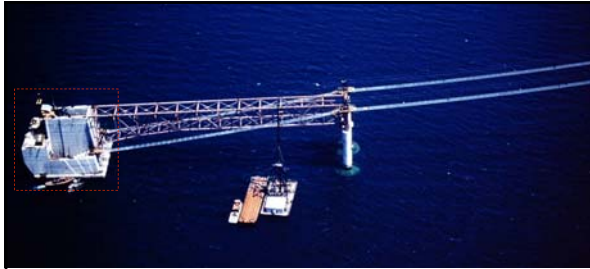
Above: caption: "Temporary catwalk in place before the start of the construction of the Mackinac Bridge cables." The anchorage is at left in photograph.
