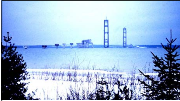
Above: caption: "Mackinac Bridge construction goes on hold during the winter of 1955-56."
