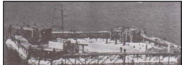
Above: caption: "As with the anchor blocks work resumed on the main tower foundations as soon as the ice melted. Notwithstanding the fears of the faint-hearted who were certain the bridge work would never stand the Straits ice, there was no ice damage whatsoever. Here is one of the incomplete caisson foundations. A twin-walled steel can without concrete reinforcing challenged the winter's worst. And when spring came. Inspection revealed that these caissons came through unscathed (Pier 19)."
