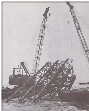
Left: caption: "Three of the four caisson corral units were lowered to overburden. Through their 20-inch pipes heavy piles were driven to rock. Concrete was pumped into the pipes for additional strength. Next, the caisson was towed into position flush against the three units of the corral already anchored. Then the fourth side was installed. Thus the huge caisson was held in position while being lowered to the bottom, despite wind and high water. All movements were directed by surveyors from triangulation towers."
