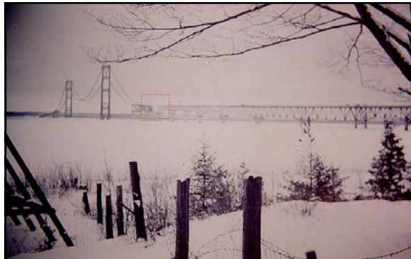
Above: caption: "As the work is suspended for the winter of 1956-57, the bridge roadway is nearly complete up to the two anchorages." 327
