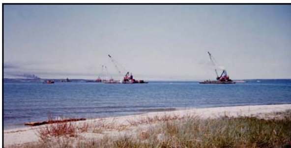
Above: caption: "Several MC&S floating cranes (on barges) at work on the construction of the piers for the south-end of the Mackinac Bridge, with Mackinac Island and Bois Blanc Island in the distance. View from southern shore."
