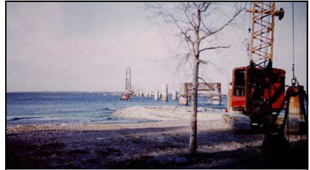
Above: caption: "Mackinac Bridge pier construction nearly complete. Note formwork for connecting beam for the pier in foreground (near shore.)"
