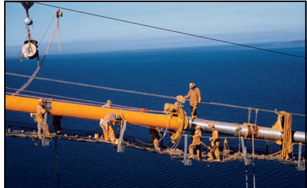
Above: caption: "While all the work on the roadway was going on, men were strung out overhead on eight sections of the cable applying red lead paste and wrapping thin steel wire as tightly as possible around the cable to provide protection against the elements." 368
