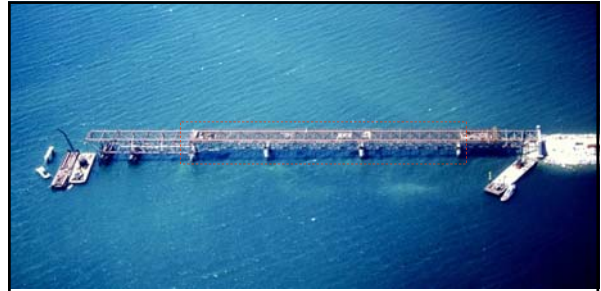
Above: caption: "Construction began from the causeway on the St. Ignace (north) side of the Straits in a southerly direction in mid-May 1956. The truss sections were floated into position then topped with the roadway stringers which can be seen atop the three center sections."
