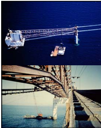
Top: caption: "Temporary catwalk in place before the start of the construction of the bridge cables. Construction of these catwalks was very hazardous and two Bridge workers fell to their deaths during their construction."
