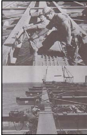
Top: caption: "Bridgemen tightening high tension steel bolts used for all truss span connections. Meter in torque wrench must be carefully observed to make sure that a bolt is neither too tight nor too loose. Every bolt was inspected."
