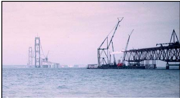
Above: caption: "A marine crane on barge preparing to raise a truss section of the framework into place." 165
