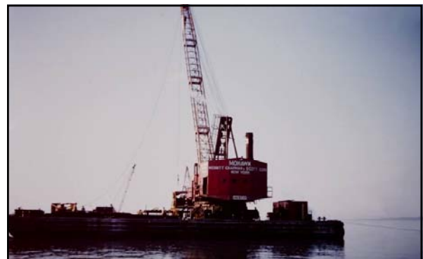
Above: caption: "An MC&S floating crane used in the construction of a Mackinac Bridge pier."
