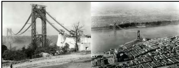
“...Less than eight days were required for the erection, without accident, of the two footbridges. During the footbridge construction the company's launch cruised continually under the bridges to immediately render aid should it be needed...”
