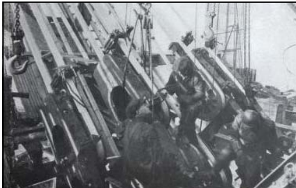
Above: caption: "Strand arms connected to anchorage eyebars. Adjusting strands at New York anchorage." 327
