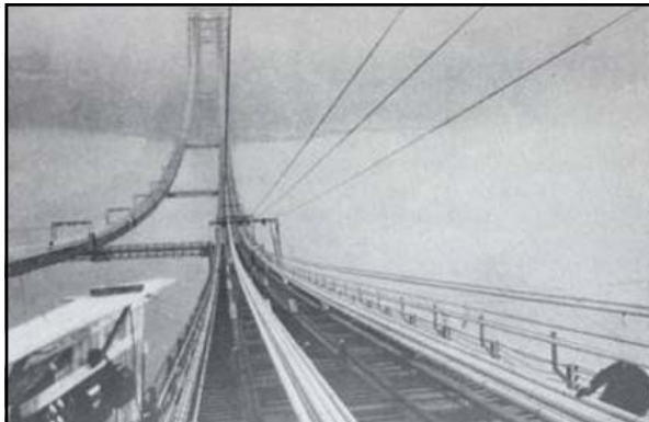
Above: caption: "Groups of strands adjusted for each of the four cables. Note ample working space on both sides of cables, spinning tramways overhead, signal wires alongside hand rails, and signal station at left" 357
