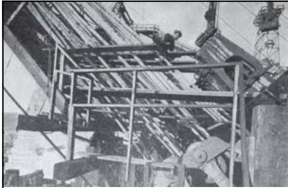
Above: caption: "Lower tiers of strands connected to eyebars in New York anchorage, and working platforms prepared for spinning higher and higher tiers of strands" 337
