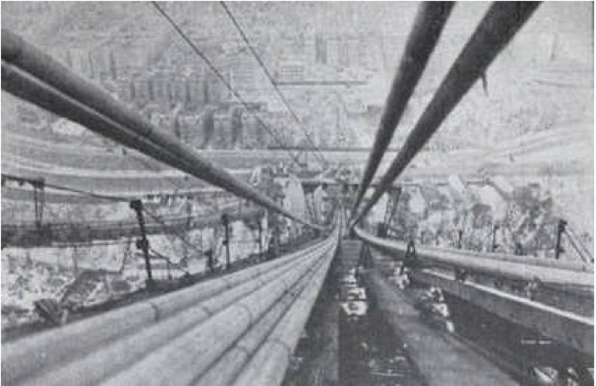
Above: caption: “Four strands completed and ready for adjustment with those already positioned in cable B”
