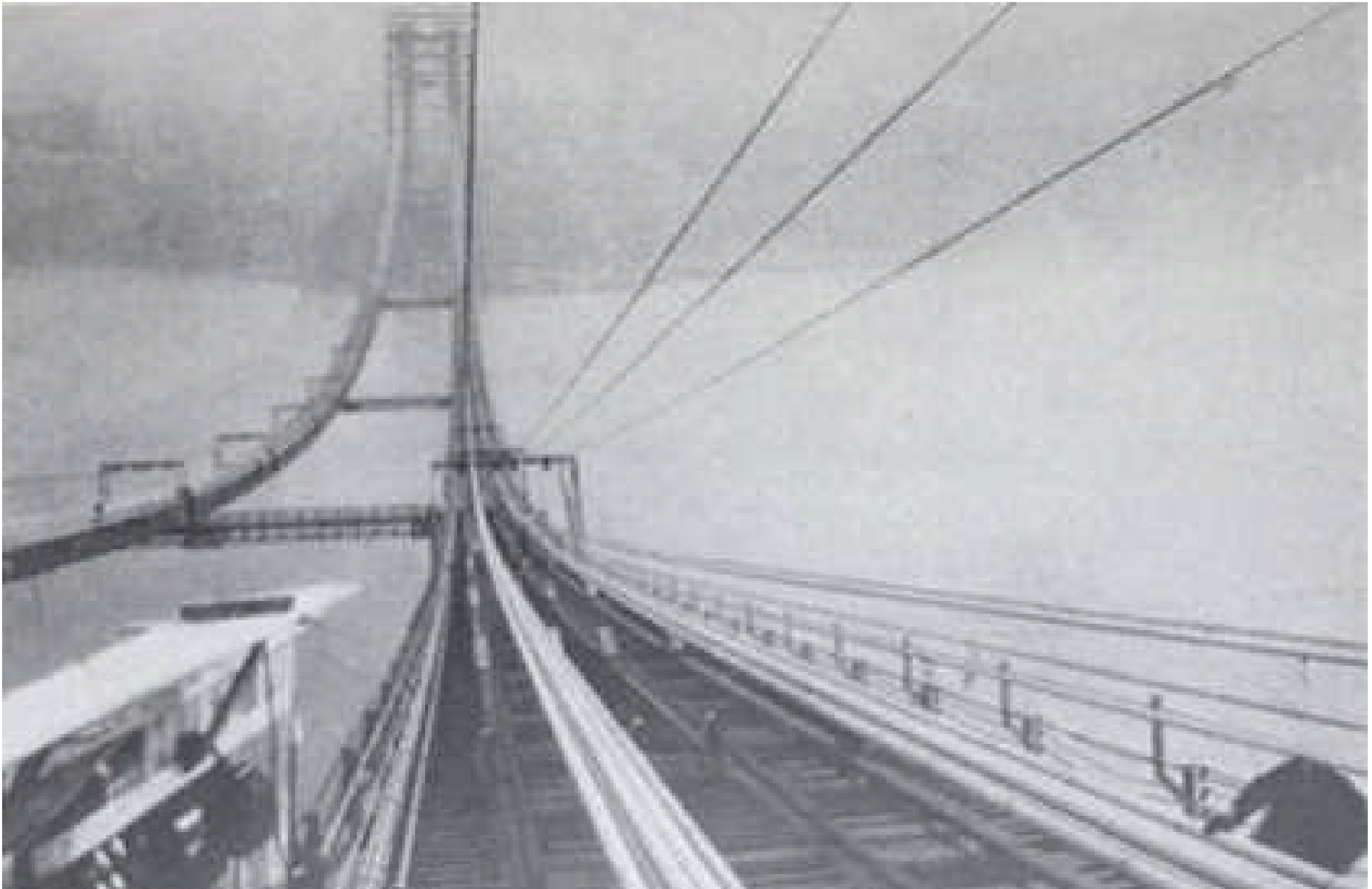
Above: caption: “Groups of strands adjusted for each of the four cables. Note ample working space on both sides of cables, spinning tramways overhead, signal wires alongside hand rails, and signal station at left”
