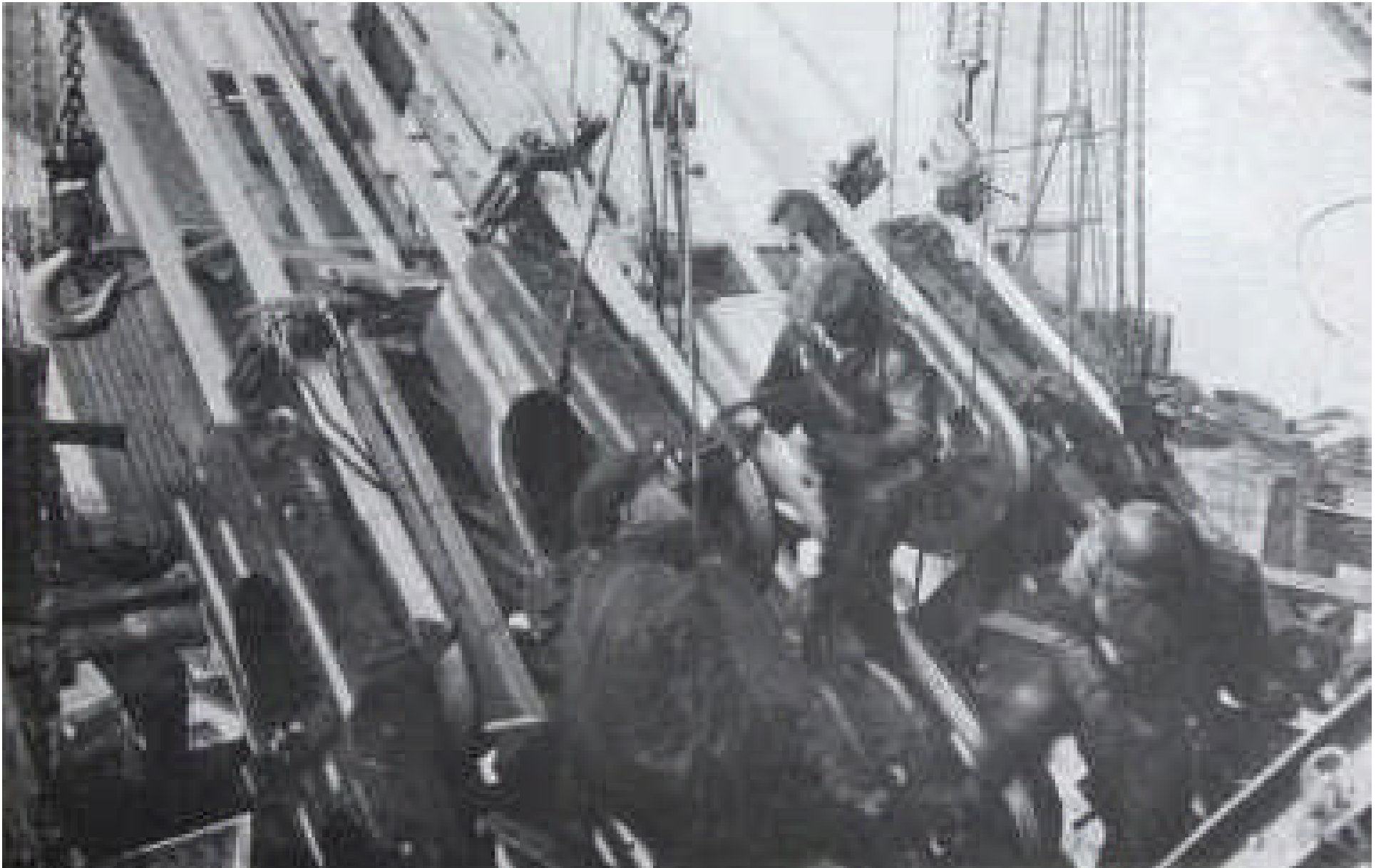
Above: caption: “Strand arms connected to anchorage eyebars. Adjusting strands at New York anchorage.”
