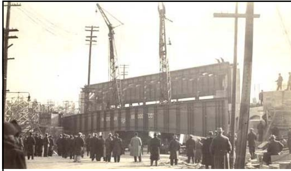
Above: caption: "Installation of the bridge carrying the Lincoln Tunnel approach over Park Avenue. Placing 55-ton steel to complete the ramp on Park Av." 103
