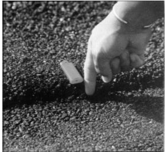
Figure 3.8. Overfilled patch area
