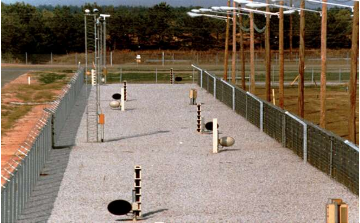
Figure 9b Double fence line
