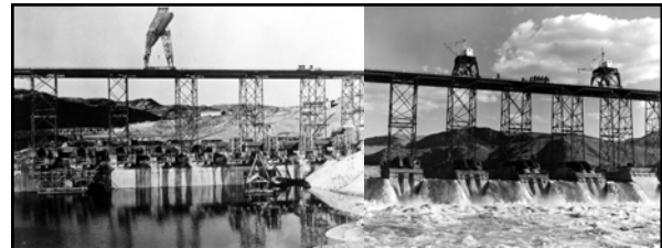
"...The CBI will place about 55,000 cubic yards in the next two months, and will then make extensive changes in equipment. The construction trestle, extending the length of the dam, will be raised about 200-feet and will be nearly doubled in width. The concrete mixing plant will be moved about 180-feet higher on the east bank. Approximately 2,000 men are employed by the Reclamation Bureau, the CBI and subcontractors at the dam site and in the Columbia basin."
