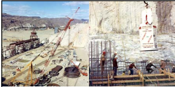
Left: caption: "October 13, 1970. Third Power Plant construction at Grand Coulee Dam." Right: caption: "October 21, 1970. First bucket of concrete for Third Power Plant."
