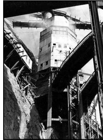
“...In the house of magic, the concrete mixing plants at either end of the dam site, are other operators who in turn cause sand and gravel to flow to their institutions over special conveyor belts. Manipulate a little gadget, and the sand and gravel falls from the bottom of the pile onto a moving belt to be rushed off to the waiting bin in the mixer plant...”
