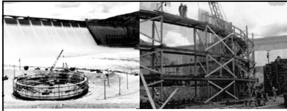
Left: caption: "Caisson graving dock where caisson will set. Caisson will be used for spillway bucket repair at Grand Coulee Dam (June 1944)"
