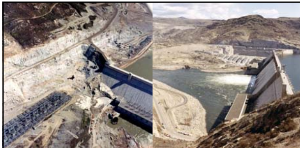
Left: caption: "April 9, 1970. Third Power Plant construction at Grand Coulee Dam." Right: caption: "May 4, 1970. Third Power Plant construction at Grand Coulee Dam."
