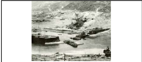
"Engineers estimate that Block 40, closest to the cofferdam, will have been poured to its contract height sometime in April. After the cross-stream cofferdams are built, the first cofferdam will be removed, and the river diverted around the excavation area over the concrete. Both ends of Block 40 will be tied in securely with the cell clusters from which the cross-stream coffer will be built..." Spokesman-Review, January 13 th 1936 1311
