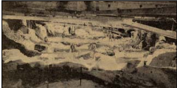
Above: caption: "MWAK workmen excavating bedrock to permit construction of Block 40 of the Grand Coulee dam. These men are working more than 70-feet below and within 100-feet of the Columbia river. At the south end of the shaft bedrock has been excavated more than 115-feet below the river level. At the north end deep rock excavation has been done in order to pour the 'bucket' or downstream toe of the Grand Coulee dam. It is expected that considerable concrete will be poured on this bedrock within the next month or six weeks." (Spokesman-Review, January 19 th 1936) 1312
