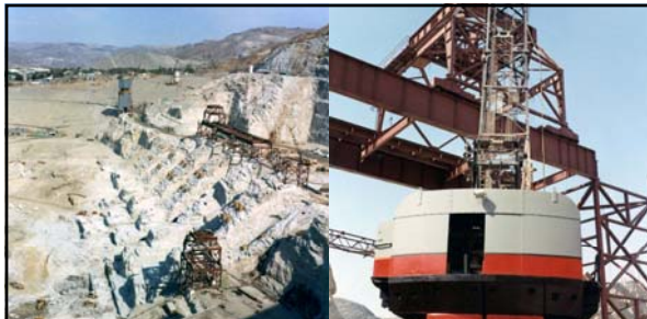
Above L&R: caption: "September 29, 1970. Third Power Plant construction at Grand Coulee Dam."
