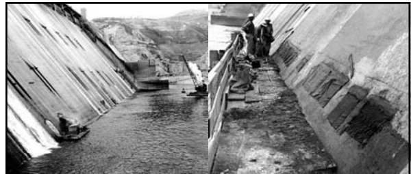
Left: caption: "Concrete being repaired on face of Grand Coulee Dam, March 1949"
