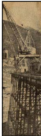
"A form-a-day seems to be the slogan of MAWK in the construction of concrete-blocks near the west abutment. Carpenters and other workmen are engaged on the fourth and largest of the forms today. This block is located against the west abutment, the other three forming a line with spaces in between toward the coffer-dam..."
