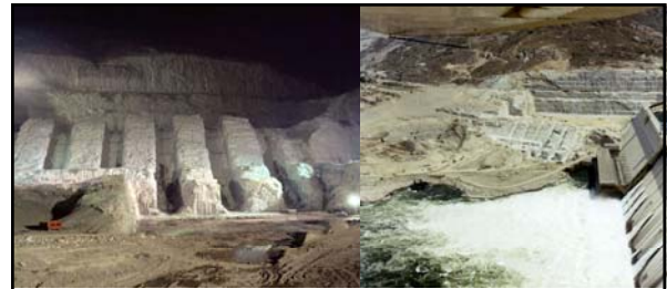
Left: caption: "May 20, 1970. Third Power Plant construction at Grand Coulee Dam." Right: caption: "May 22, 1970. Third Power Plant construction at Grand Coulee Dam."
