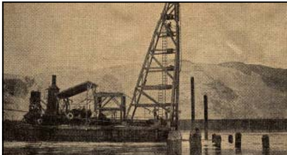
Above: caption: "MWAK engineers accomplished a difficult feat in building a conveyor belt across the Columbia river at the Grand Coulee dam. The work is almost completed. The picture shows the pile-driver mounted on a barge, in operation over a portion of the river 60-feet deep. The current was so strong that 18-inch fir piling snapped off. The engineers then tested driving steel I-beams, but the current twisted them into spirals. MWAK then ordered from the coast the longest piling available, 130 to 140-foot lengths cut off the slender ends, lashed the pilings together in groups of three, and drove them successfully. The dock is being built on the trestle, which will soon be in use conveying dirt from the east bank excavation to the conveyor on the west bank, which will dump it in Rattlesnake canyon." (Spokesman-Review, August 17 th 1935)
