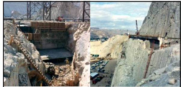
Left: caption: "September 29, 1970. Third Power Plant construction at Grand Coulee Dam." Right: caption: "October 9, 1970. Third Power Plant construction at Grand Coulee Dam"
