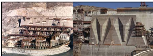
Left: caption: "February 21, 1973. Third Power Plant construction at Grand Coulee Dam." Right: caption: "May 5, 1973. Third Power Plant construction at Grand Coulee Dam."
