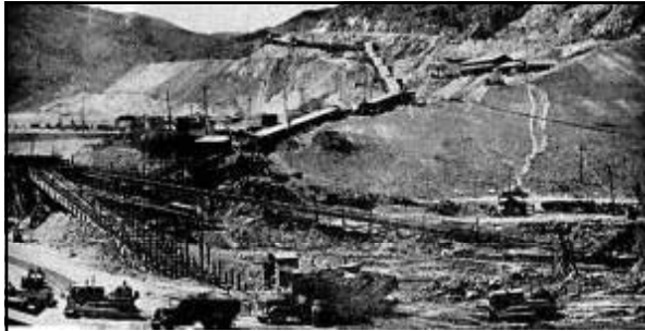
Above: caption: "Digging a 35-Acre Hole to Bedrock. To remove the 44 million tons of earth and rock from Grand Coulee Dam site, a conveyor belt was laid which, fed by a fleet of tractors and buggies, carried all but the large rock a mile and a half over the hill to Rattlesnake canyon on the west side of the river. Material excavated on the east side journeyed across a conveyor bridge and made connections with the Rattlesnake Express. For four years this conveyor operated." 565
