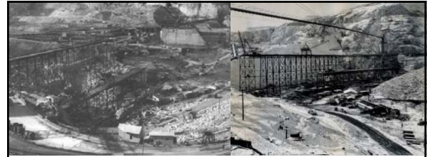
Left: caption: "This is the dam as it looked in late 1936 from the river's east bank. Trestles in the left foreground mark the present line of the dam. The area is enclosed by a cofferdam and the river is flowing through the partially completed section of the dam in the upper right of the picture." Right: caption: "Construction of Grand Coulee Dam, ca. 1936"
