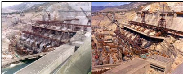
Left: caption: "June 10, 1971. Third Power Plant construction at Grand Coulee Dam." Right: caption: "August 1, 1971. Third Power Plant construction at Grand Coulee Dam."
