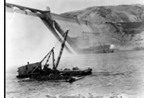
Bottom: caption: "Excavating river bottom prior to setting up caisson for spillway bucket repairs at Grand Coulee Dam (January 1947)"
