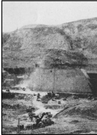
"...Most of this material has been moved one and a half miles away by conveyor belts where it filled a convenient ravine. Today the conveyor belts have reversed their direction and are bringing endless streams of materials down out of the hills to the concrete mixers..."
