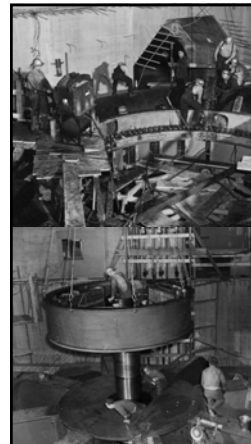
Top: caption: "Riveting together the sections of the No. 1 Shasta turbine scroll case in pit 7. This unit consists of several radial and on straight section of welded plate steel riveted with double butt straps. Before being poured in concrete, the scroll case is given hydraulic test of 310 psi. This scroll case, designed for use at Shasta Dam in northern California, is temporarily installed at Grand Coulee Dam by order of the War Production Board, as construction at Shasta Dam had not progressed sufficiently to make immediate use of turbine at that point. With the waters of the mighty Columbia River as a driving force, this turbine now installed is spinning a giant generator at a rate of 138.5 rpm, producing more than 75,000 kilowatts of electrical energy, Feb. 1942"
