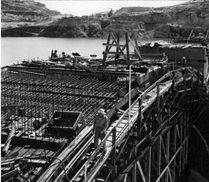
Top Left : caption: “View of the spillway section from the left bank, February 1941”
