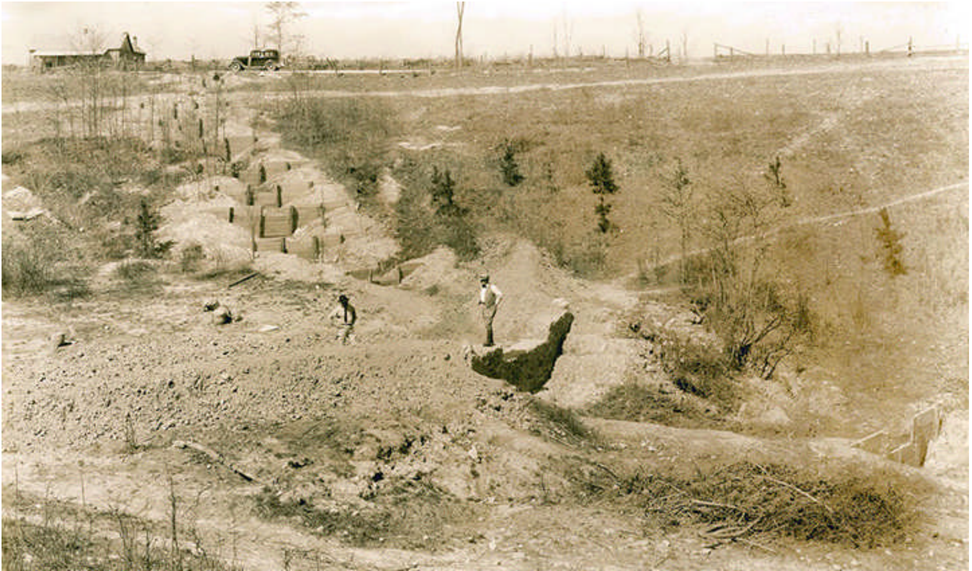
Above: caption: “CCC Tennessee Soil Erosion Project. “Improper disposal of the drainage from the highway caused the erosion in the head of a farm near Demoray. Plank check dams were built in the main gully, with a masonry soil-saving dam constructed at a point where it would catch a considerable amount of silt. The further treatment of this area will be to plant locust and pine.”
