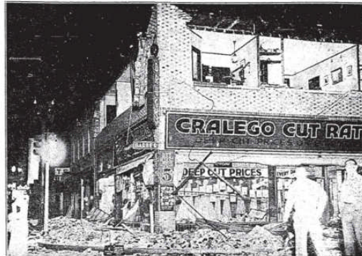
Southeast Corner Florence and Compton Avenues, where upper half of building fell out. —Corbett Photo Service.
