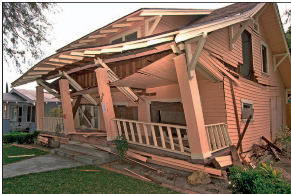
Figure 15-6. A house with severe damage due to cripple wall failure
