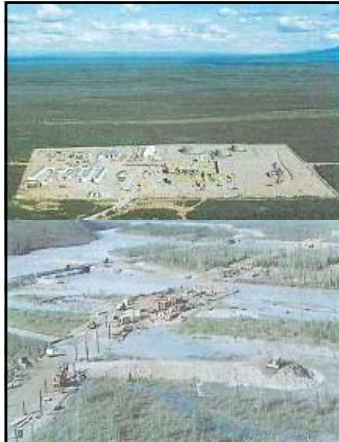
Left: caption: "Plate 28. Pump Station 9 which was constructed in spruce-deciduous woodland (HMQ) and spruce woodland (LMQ) in A.S. 44, Section 2. View is east. The work pad joins the north and south sides of the site (about 43 acres). June, 1977." Bottom: caption: "Plate 24. Spur dike construction (dozer on 'nose' of dike) and river-crossing staging area on the Hammond River, A.S. 101, Section 5. The pipeline crosses the Middle Fork Koyukuk River in the upper right corner of the photo. View is north. Haul Road is to the west of the pipeline. June, 1976." 577
