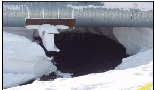
Above: caption: "March 2, 2006: A worker at Prudhoe Bay spots the frozen tundra drenched with some 200,000 gallons of oil. Unbeknownst to BP, one of the company's transit pipelines had become corroded and was leaking for days, resulting in the biggest spill ever recorded in an Alaska oil field. A pipeline detection system failed to catch the leak."
