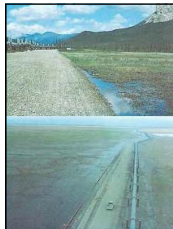
Top: caption: "Plate 19. Work pad and elevated pipeline built through wetlands (HQ) in A.S. 103, Section 5. View is north. Cross-drainage is from east to west; note ponding on right side of pad. June, 1977." Bottom: caption: "Plate 20. A section of work pad through wet-meadow tundra (HQ) in A.S. 137, Section 6. View is north. The fuel gasoline can be seen on the west side of the pad with the 48" pipeline on the right side. Both segments of pipe are resting on wooden cribs prior to installation. Note ponding on west side of pad throughout photo. June, 1976." 582
