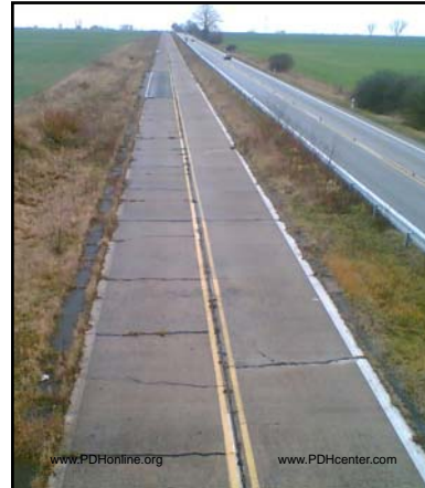
"...Newspaper the Welt am Sonntag reported that the road survived Nazism and Communism and despite some repair work is still the original stretch from the 1930s. But drivers have had enough of the cracks and potholes on the route which links Berlin to the Polish city of Szczecin. Frank Götzmann, director of the nearby town of Gartz, told the newspaper: 'The condition of the motorway is unbearable. Everyone drives carefully on it'..." theLocal.de, Sept. 2013
