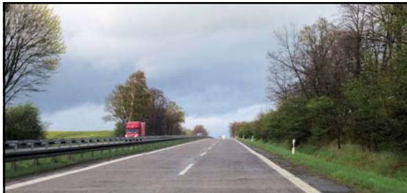
"...In 2016 the road will be 80 years old, so 'maybe Unesco will make it a world heritage site,' he joked. The road was laid using 25-metre-long concrete slabs. These are cracking under the weight of the traffic as well as the weather. But Arndt said the stretch of road was his favorite because of the history and the countryside, the Welt am Sonntag reported. Renovation is planned for 2015 if the money can be found. Five bridges on the A11 also need rebuilding which date from the 1930s."
