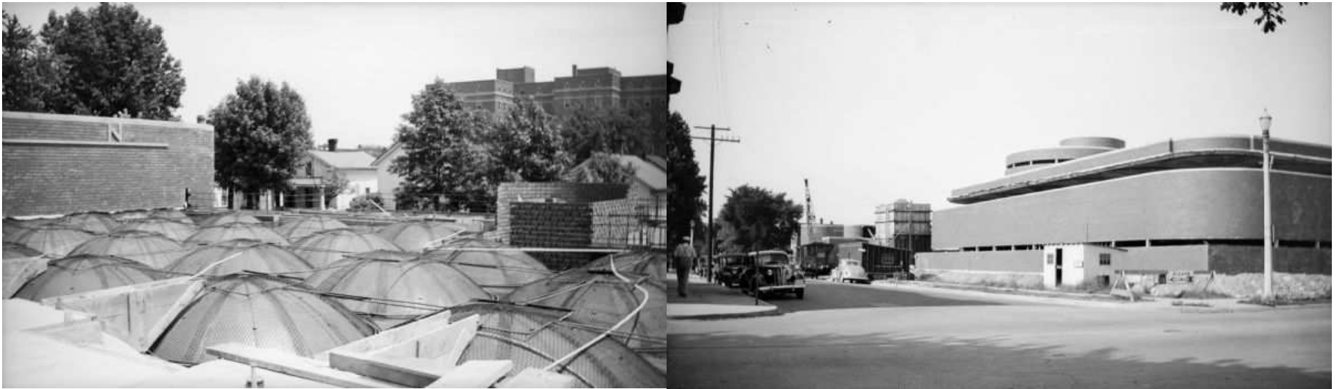
Above Left: caption: “Roof of the Johnson Wax Administration Building during construction. The skylight domes have been installed.”
