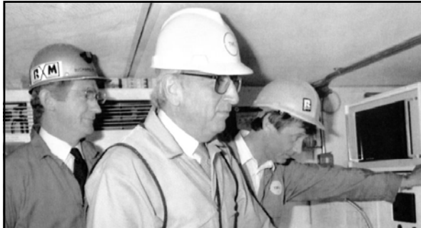
Above: caption: "Trade and Industry Secretary Lord Young (centre) presses the start button on the tunnel boring machine in the south marine running tunnel at Dover, watched in by Richard Lewis (left), of the machine's manufacturer, Robins Markham. May 6, 1989." 1225
