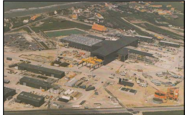
Above: caption: “Aerial View of Sangatte Construction Site, June 1988. The main shaft for tunnel construction is under the building complex in the center of this picture.”
