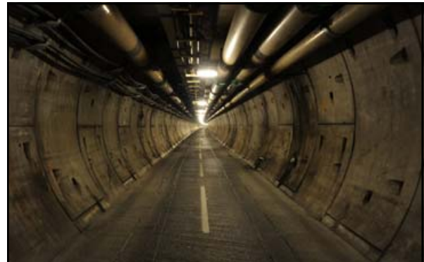
The service tunnel is 4.8-meters in diameter and lies between the two rail tunnels (15-meters away from each of them). In normal operations, shuttles use the south tunnel in the France-to-UK direction and the north tunnel when travelling from the UK-to-France. A vehicle was specifically designed for travel in the service tunnel. It's multi-functional and is used for maintenance operations and in case of incidents, with the aim of reaching the scene of an incident in minimum time.
