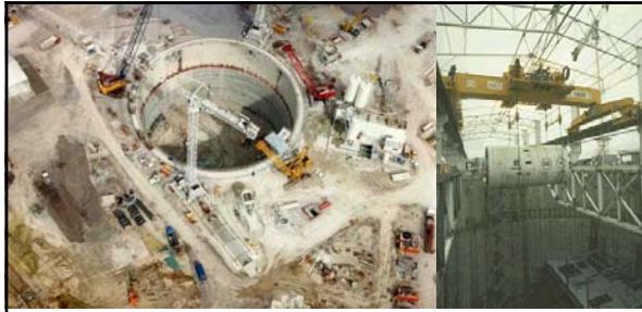
In order to excavate the tunnel, an access shaft was constructed in Sangatte. Due to the presence of an aquifer, the access shaft was built inside a waterproof form. Measuring 55-meters in diameter and 75-meters high (the volume of excavated material was 390K cubic-meters), it allowed TBMs to be lowered and assembled under dry conditions. Left: caption: "After completion of the construction phase, the well will house the ventilation facilities and other essential services" Right: caption: "Lowering TBM via access shaft"
