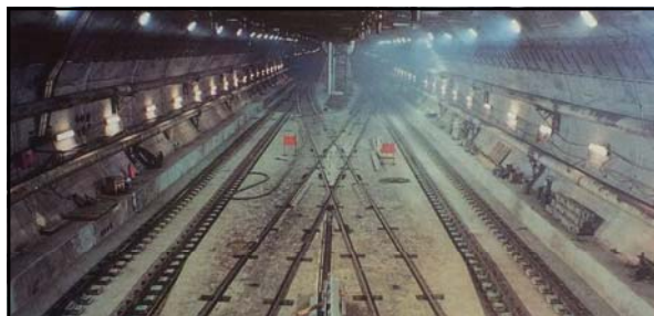
The French crossover is located 12km off the French coast in less favorable ground conditions. The chamber was constructed using a series of contiguous small diameter tunnels with a minimum height of 2-meters and has overall dimensions of; 180-meters-long, 19-meters-high and 25-meters wide. Above: caption: "Channel Tunnel Project – December 18, 1992: the development of the French Crossover is complete. An equivalent structure was built on the British side." 1595
