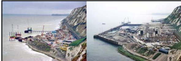
Left: caption: "Channel Tunnel work site seen from Shakespeare Cliff in January 1989. Channel Tunnel works begin. The first step is to greatly enlarge the land area by driving steel sheets into the sea bed to make a coffer dam. This was subsequently filled with concrete. Then the enclosed area pumped out and filled with sand."
