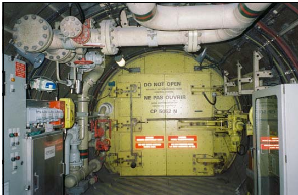
Above: caption: "The communication gates between the service and rail tunnel can be controlled manually within the tunnels or from the Railway Control Centre (RCC)"
