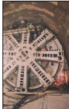
"...Back in bore position finally, the massive cutting disc begins to rotate, slowly revving to its maximum of 3.3 rpm. It grinds out the chalk in fist-size hunks that are scooped up and dumped onto a conveyor leading through the TBM's innards to its rear. There, in a dust bowl of swirling grit, the chalk dumps into small boxcars to be shuttled off..." Popular Science, June 1990
