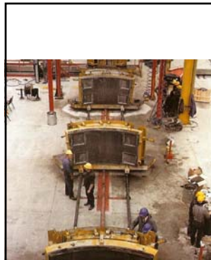
"...Later, the grouting crew, wielding fire hoses of mortar, fills any gaps between plates. They inject the mixture under pressure, squirting it between the sheathing and rock - and often onto themselves. It seeps into rock cracks, strengthening and forming a barrier. 'It's a nasty job,' one of the workers told me later. 'It's especially bad when you're working overhead - the worst job down there..." Popular Science, June 1990
