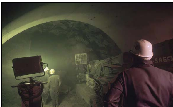
Above: caption: "Sangatte, France. July 27, 1987: At the bottom of a 55m diameter and 60m deep vertical well, 450 workmen took turns night and day. Eleven specially built tunnel borers (six British and five French) made it possible to advance up to 500m a month"
