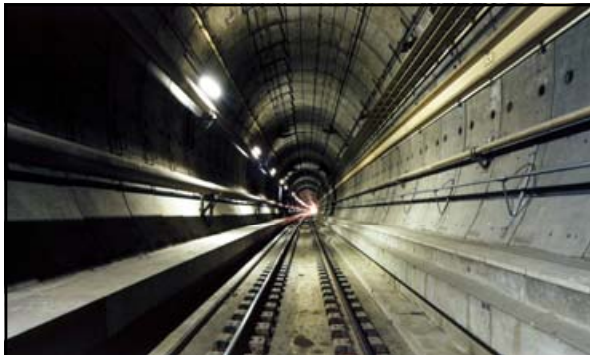
The two rail (a/k/a "running") tunnels are 7.6-meters in diameter and 30-meters apart. Each rail tunnel has a single track, overhead line equipment (catenary) and two walkways (one for maintenance purposes and the other for use in the event of an emergency evacuation and on the side nearest the service tunnel). The walkways are also designed to maintain a shuttle upright and in a straight line of travel in the event of a derailment. The track in each rail tunnel has two continuously welded rails laid on pre-cast concrete supports embedded in the concrete track bed.
