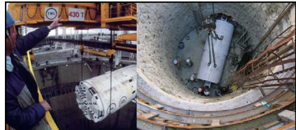
"...This mole - nowadays they call them TBMs, tunnel-boring machines - was built by Scotland's James Howden & Co. Others, of various styles, were designed jointly by The Robbins Co. of Kent, Wash., Markham & Co. of Chesterfield, England, and Komatsu Ltd. And Kawasaki Heavy Industries Ltd. in Japan. In both England and France, the TBMs were lowered down access shafts in massive hunks, then assembled at tunnel level..."
