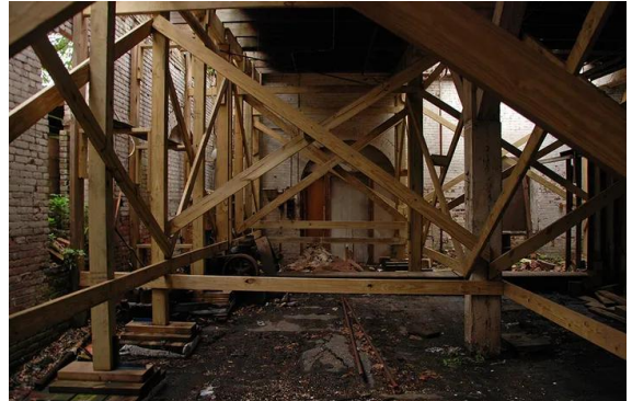
1556 Caption: "The interior of the shed is being supported by a forest of wooden braces. In its previous life, the structure was used to dry-out the masts of boats built in the Navy Yard."
