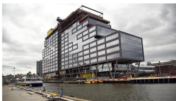
"...This new office tower, which topped out last October, will house a 220,000 square-foot WeWork facility. It's built out onto a narrow dock located between Dry Docks 2 and 3, which are controlled by the BNYDC, and currently flooded and inactive..." ny.curbed.com, May 3, 2018
