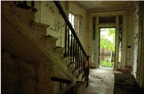
Caption: "Some building interiors are still in relatively good condition, despite being exposed to the elements for decades. The entryway of Quarters D still has stairs, floors, moldings, and windows somewhat intact."
