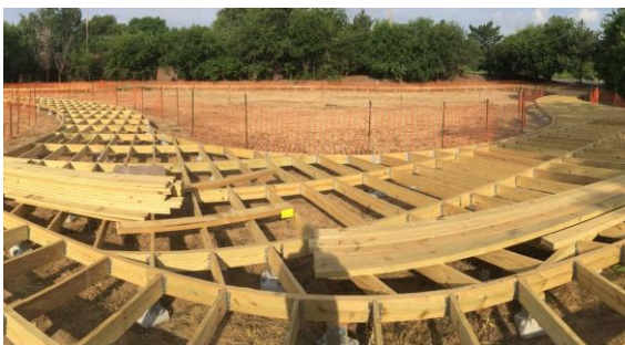
"...The walkway does not use heavy footings or foundations. Instead, an array small, precast concrete piers is set onto the ground surface and secured with steel pins driven into the earth..."
