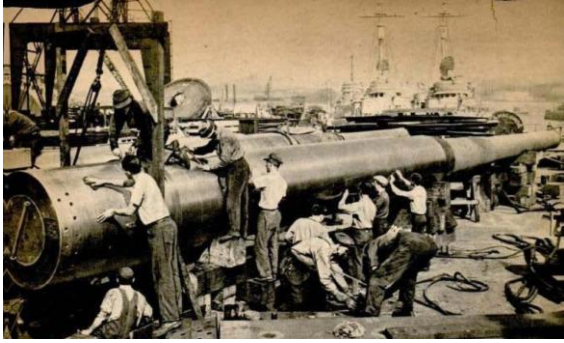
"...The crane will handle up to 900,000 pounds and it can sling a 200-ton tug, a 16-inch gun or a 150-ton turret section as a routine job..." Popular Mechanics , September 1945 Caption: "Workmen polish-up a 16-inch rifle before 175-ton crane hoists it aboard the 45,000-ton battleship Iowa"
