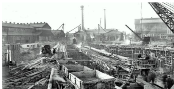
The location and orientation of the new docks was fixed within narrow limits by considerations of direct access, and by the requirements that the approach to old Dry Dock No. 4 (which lay at right angles to the new docks) be kept clear. The situation necessitated extensive dredging of existing land, filling of water areas and removal of the causeway, the two cruiser piers and all the structures on the Marine Channel. 294
