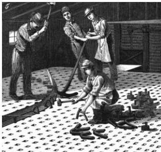
In Fig. 5, four men are bending an angle bar on the slab, a work requiring a quick eye and a ready hand, for, as is immediately obvious, the quicker the bar is bent the easier, because it stiffens as it cools. As will be seen, two men are prying with a lever, a third one hammering the piece into place, while, as the shank answers to the force, a fourth man puts in the restraining pins 955 along the chalk line already marked.
