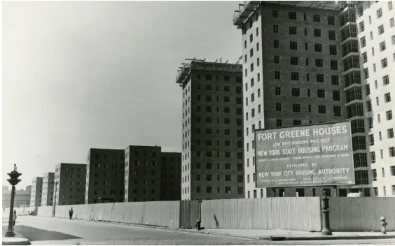
"...Work was started on the project April 14, 1941, but has been considerably delayed because of priorities. The site is bounded by Flushing Avenue, Park Ave., Tillary St., Prince St., Myrtle Ave. and Carlton Ave." 1585 The Brooklyn Daily Eagle , August 4, 1942
