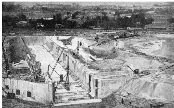
Caption: “WORK IN PROGRESS on the huge basin of the King George V Dock at Southampton. From the site of the dock about 1,258,000 cubic-yards of material were removed. The material was composed mainly of gravel which was used in making the concrete walls and floor of the dock.”
