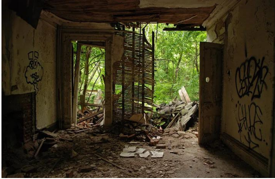
Caption: "The back-end of this building has sheared-off into the woods. Few pieces of graffiti can be found inside the buildings, which have largely been untouched by humans in 40 years, providing a case study in urban entropy." 1531
