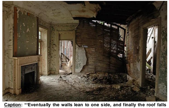
Caption: "'Eventually the walls lean to one side, and finally the roof falls in,' writes Weisman. 'Your house lasts maybe 50 years; 100, tops.' After 40 years of abandonment, many of the Admiral's Row homes appear to be near collapse." 1534
