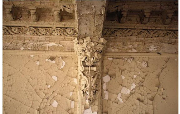
1558 Caption: "An interior view of Quarters B from 2008, revealing some of the architectural details that remained. This will be the last residential building left standing on the row."
