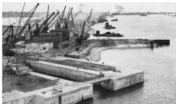
Caption: “THE CAISSON ‘CAMBER,’ or cavity, of the King George V Graving Dock, at Southampton, was excavated at the eastern side of the dock entrance. The dock is closed by a huge steel caisson. To open the dock the caisson is moved into the camber along steel runways. In the background is the line of the new quay wall and embankment which has reclaimed a considerable area from the sea and has added nearly 7,500-feet to the length of quays at Southampton.”
