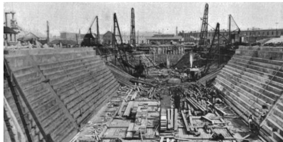
The concrete monolith will be extended entirely around the dock to the inner of the two grooves provided for receiving the caisson gate. Here the timber groove will be replaced by one in granite. It is fortunate for these repairs that the dock was designed with outer and inner grooves, since by placing the caisson at the outer groove and shoring it from the floor of the dock, as shown in one of our first page illustrations, it was possible to build the new granite groove without any further preparation.
