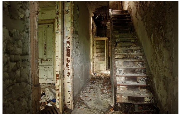
Caption: "Peeling paint, floors with holes, and crooked doorways are some of the lesser problems found inside the houses today. Feral cats, birds, and other wildlife have made them their home."
