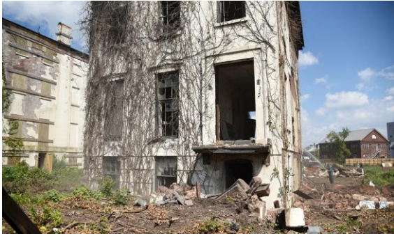
1543 Caption: "This past Friday, as workers began demolishing Building D, an enormous cloud of century-old dust and debris was released over Flushing Avenue. An inspector from the NYC Department of Environmental Protection (DEP) quickly arrived on the scene to shut-down the demolition. 'You can't knock it down that fast,' he told the workers."
