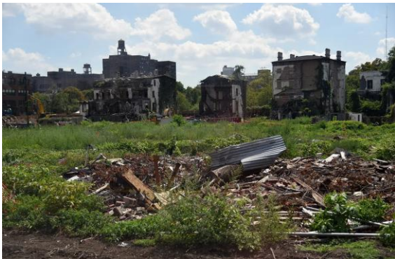
Caption: “By the end of last week, demolition was in full gear at Admiral’s Row , and by the weekend, Building D, the residence in the center, would be completely leveled by a demolition crew”
