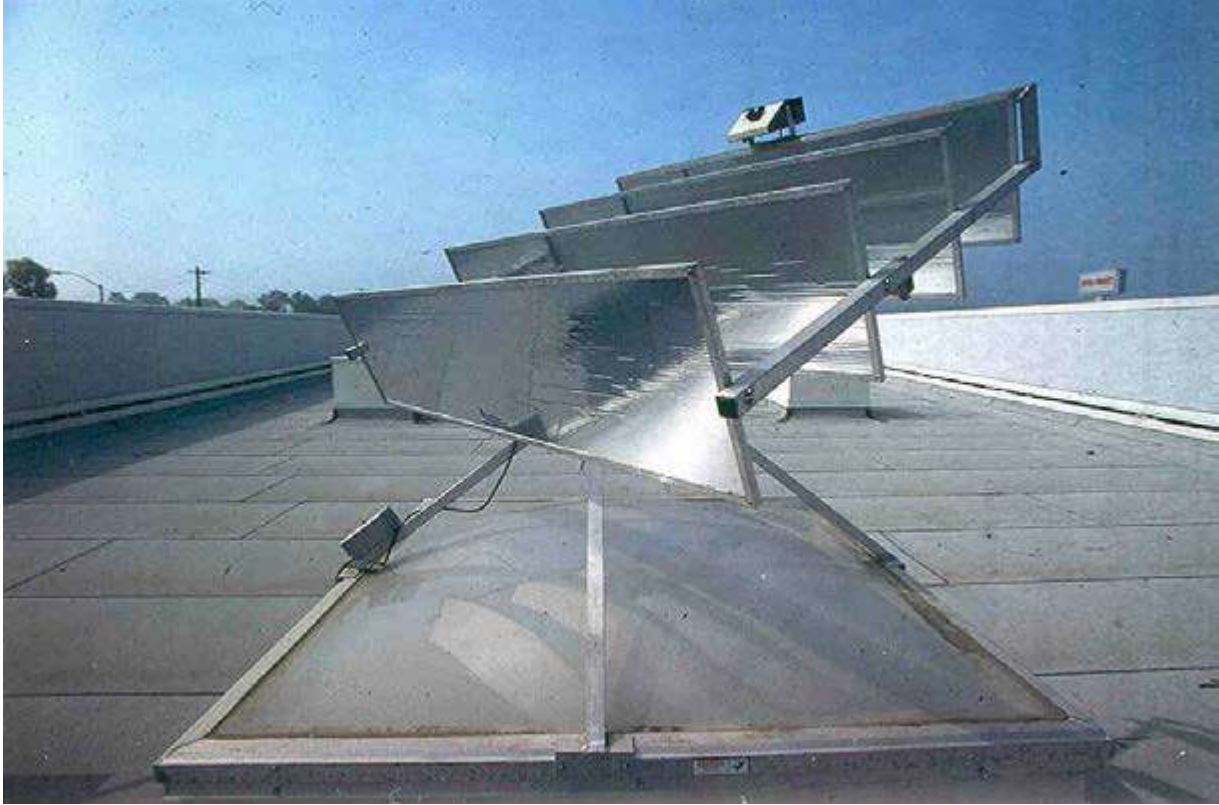
Figure 16 Example of an Active Daylighting System that Tracks the Sun and Directs Daylight into the Building.
