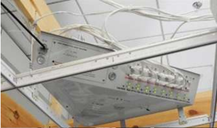
Power server module mounted above ceiling grid
