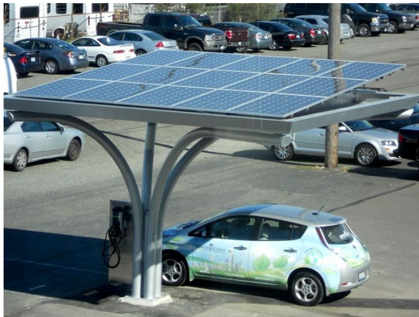
Solar Charge Station
