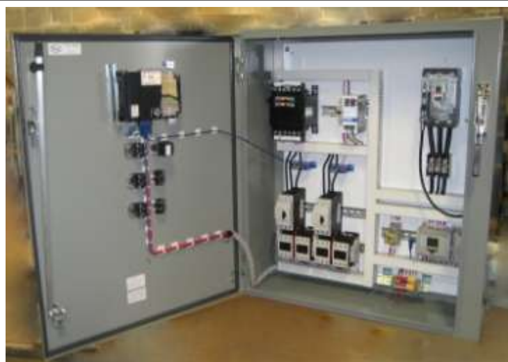
Fig. 12 - NEMA 12 Enclosure with Motor Controls
