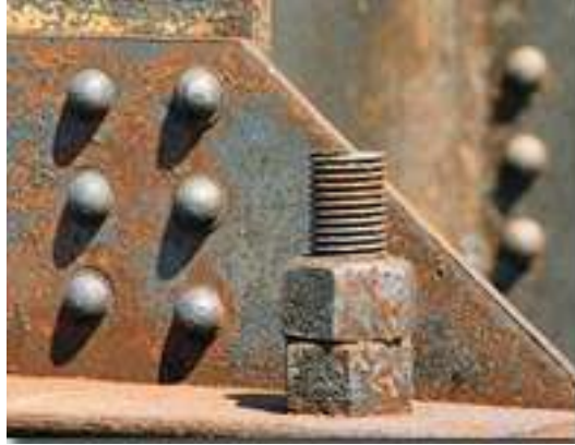
Unprotected steel will begin to corrode immediately once exposed to environment
