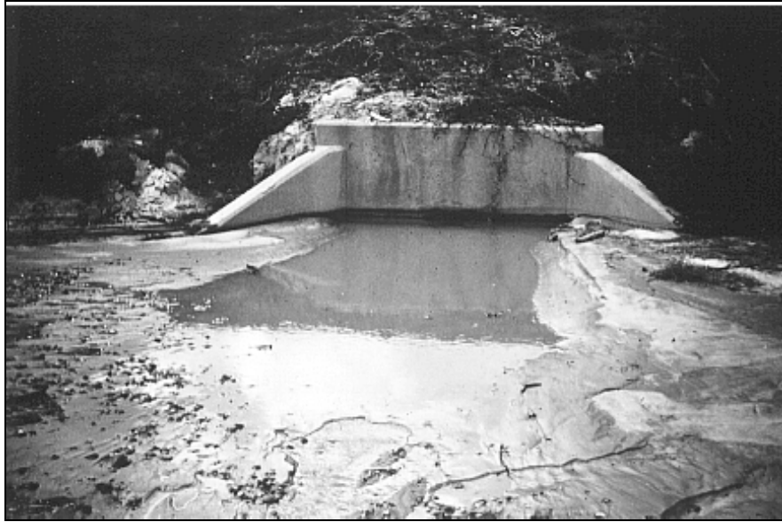
Figure VI-15--Sediment Deposition in Culvert
