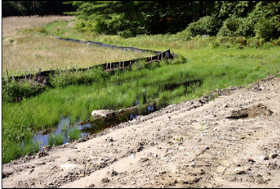
Figure 11. Illegal fill in a wetland meadow. The owner was required to remove it and restore the wetland. Silt fencing has been installed to protect existing wetlands from further impacts.
