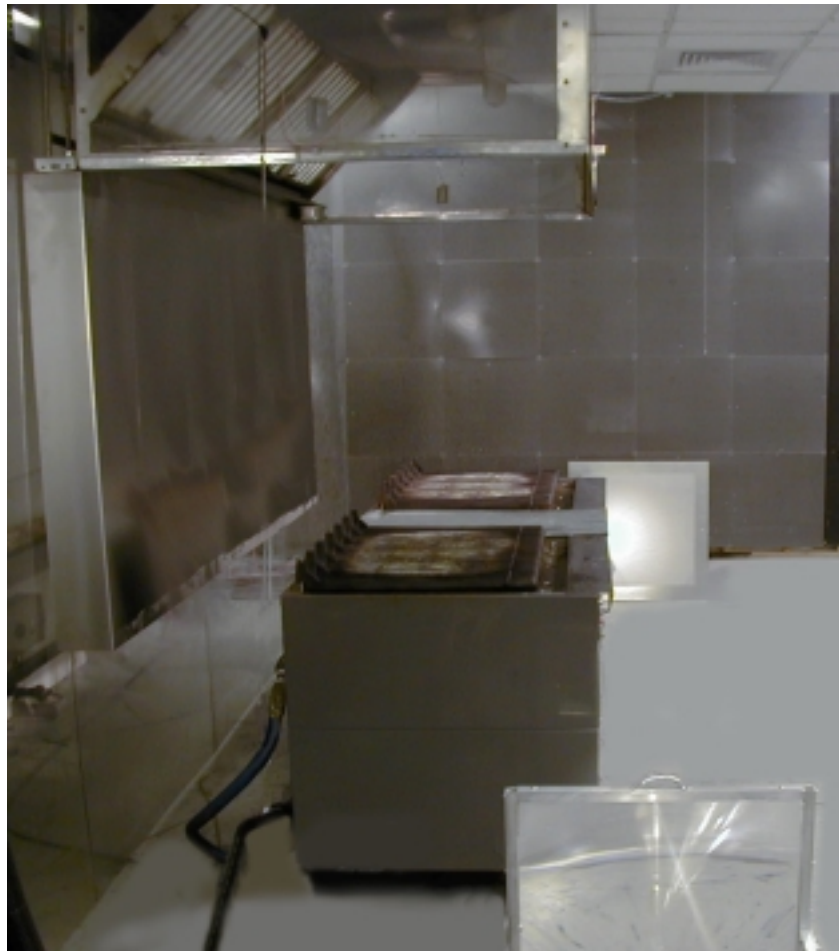
Figure 80: View of Two Charbroilers under a Wall Mounted Backwall Supplied Canopy Hood from the Perspective of the Schlieren Visualization System
