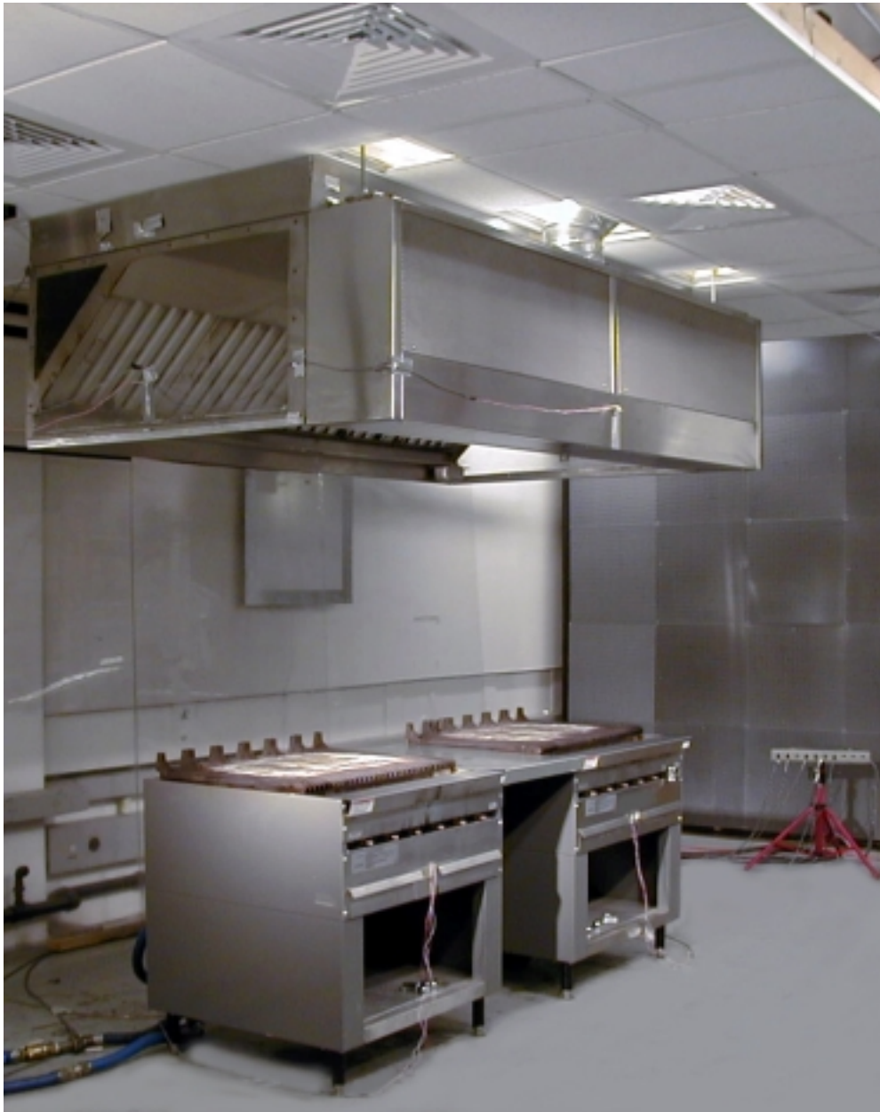
Figure 7: Two Gas Charbroilers under an 8' Hood Canopy Hood with Attached MUA Plenum with Front Face Supply
