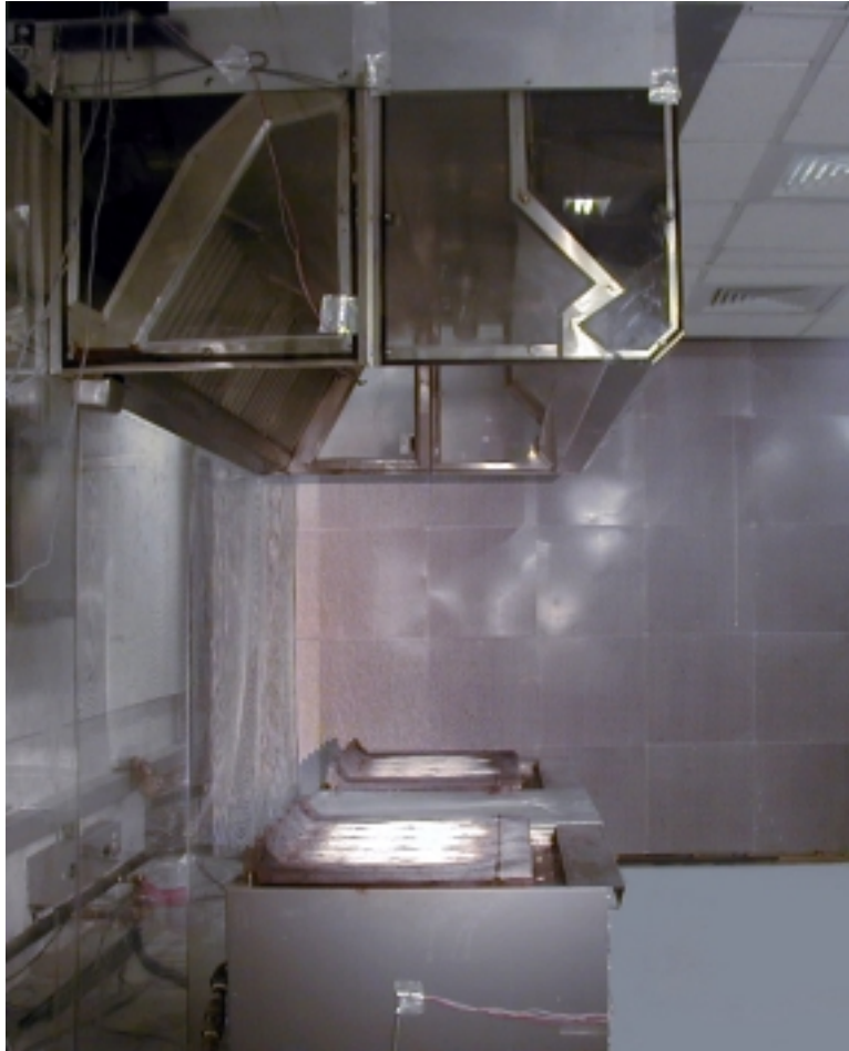
Figure 73: View of Two Charbroilers under a Wall Mounted Short Circuit Canopy Hood from the Perspective of the Schlieren Flow Visualization System
