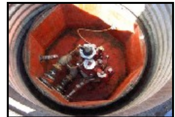
Contained turbine sump
