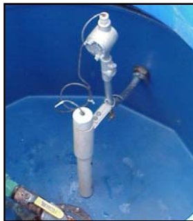
Float sump sensor
