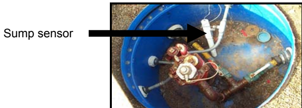
Sump sensor in contained turbine sump
