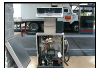
Dispenser cover pulled off to show the dispenser piping and equipment
