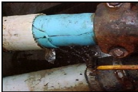
Flexible piping is cracked
