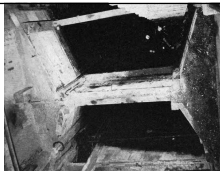
Above water-line portion of a bulkhead between the Main and Promenade Deck/s. All such bulkheads were constructed underwater by divers. 760
