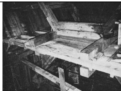
Bulkhead barrier construction at Frame 204 – Main to D-Deck (after dewatering and righting)
