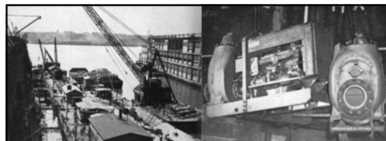
Left: derrick placing 10-inch salvage pump adjacent to Promenade Deck where rigging crews could juggle it into position once inside the ship Right: close-up of 10-inch salvage pump
